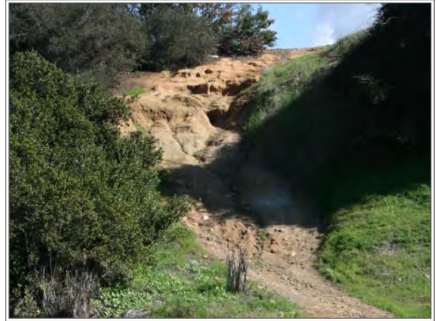
Erosion at a canyon edge
