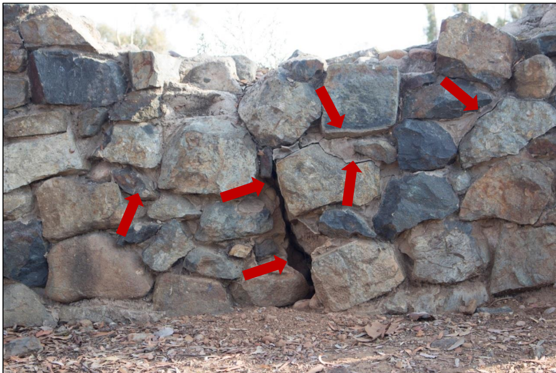
Figure 7. Detail view of wall section showing missing portions and cracks (red arrows).
