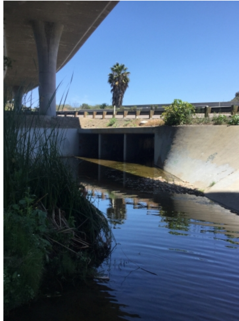
Photo 13: Downstream end of 11'x8' triple box culvert underneath Interstate 8 onramp from Waring Road
