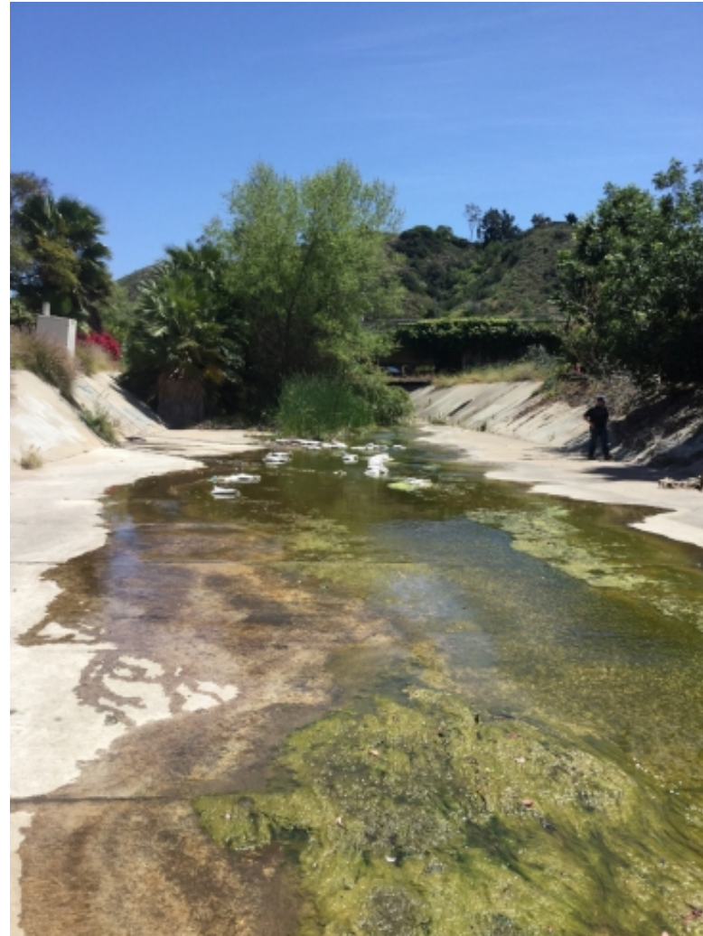
Photo 10: Bottom of Reach 5 looking upstream (W) from upstream end of triple box culvert
