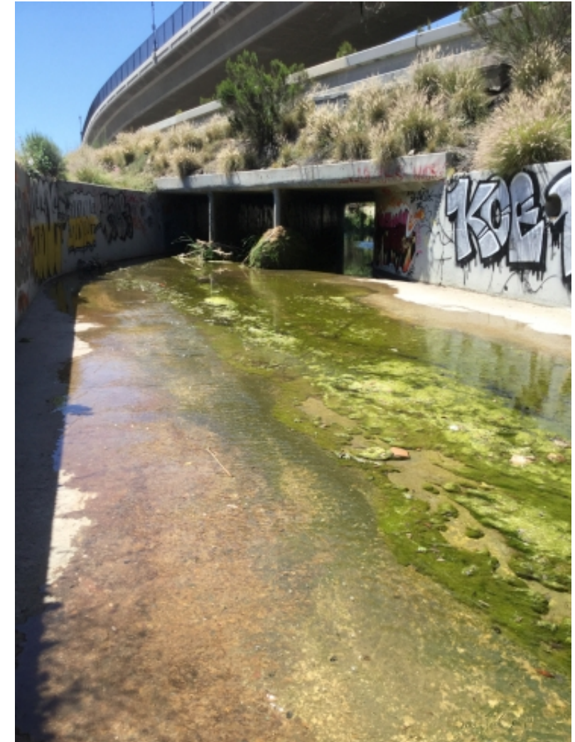
Photo 14: Upstream end of triple box culvert underneath Interstate 8 onramp from Waring Road
