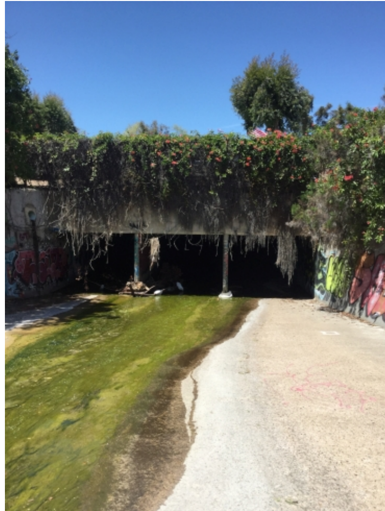
Photo 9: Looking west towards upstream end of triple box culvert from the downstream end of Reach 5
