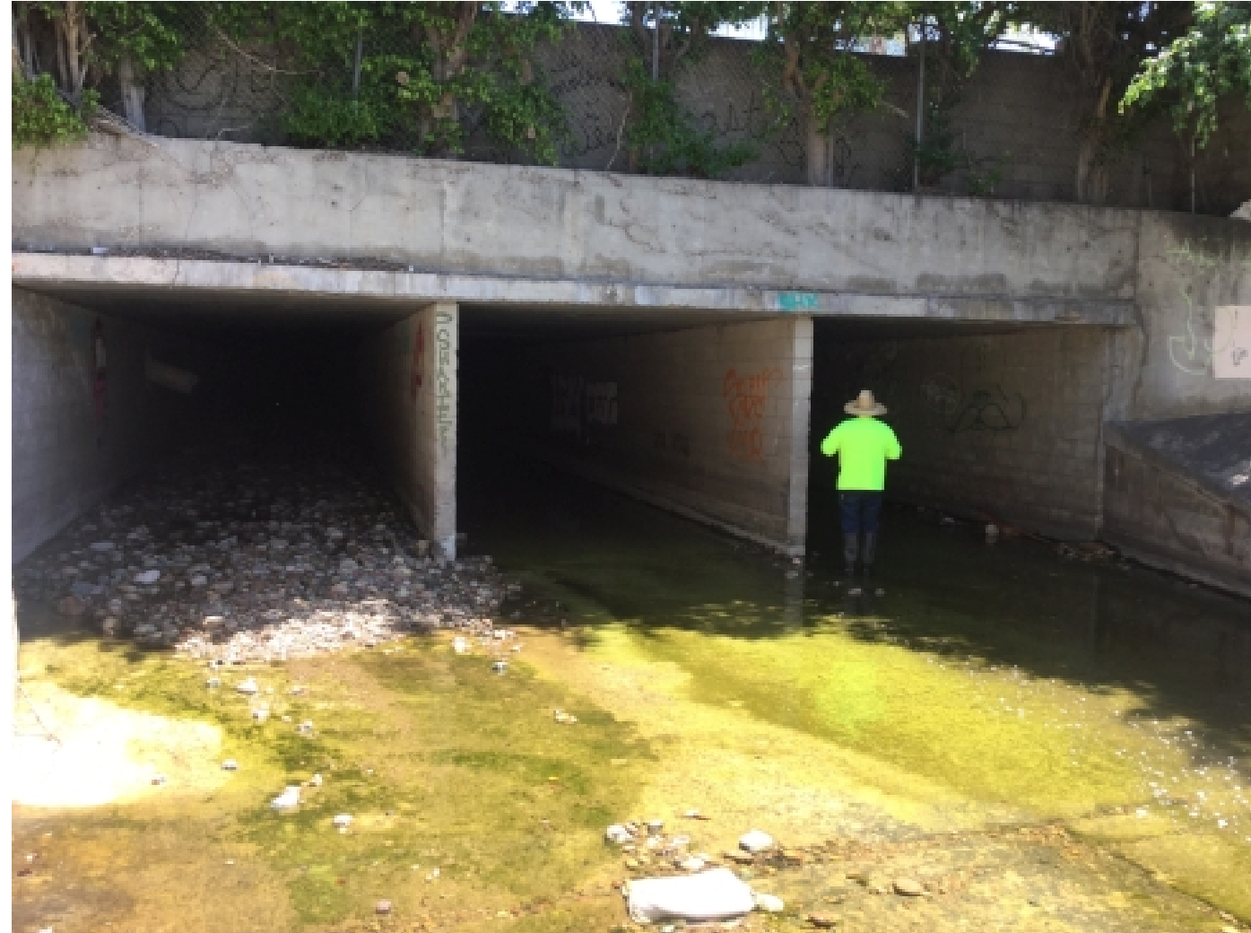
Photo 8: Close up of downstream end of 11'x8' triple box culvert underneath Grantville Business District (Reach 4)
