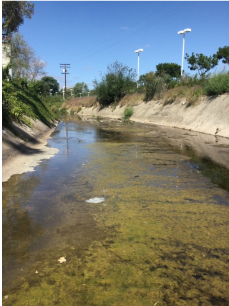
Photo 1: Looking downstream (W) from 11'x8' triple box culvert underneath Mission Gorge Road in Reach 1
