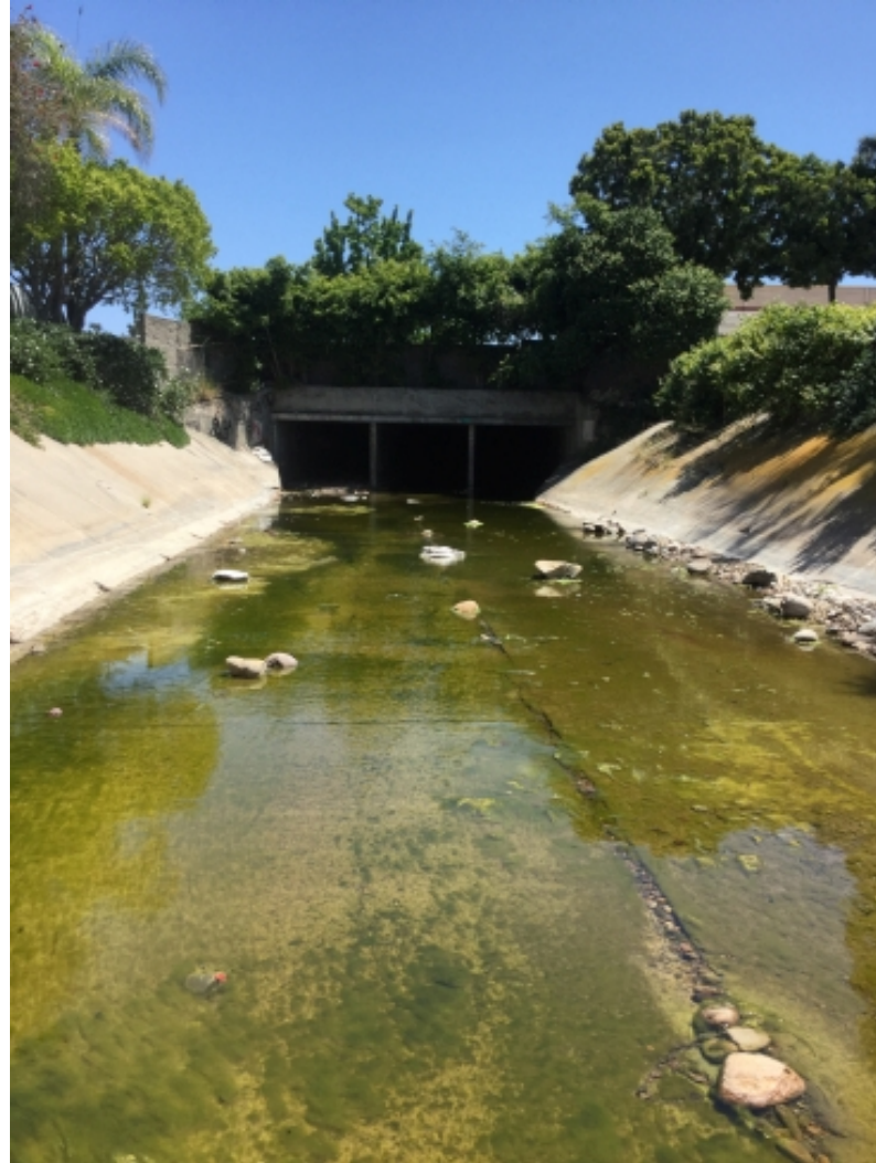
Photo 7: Reach 3 looking upstream (E) towards 11'x8' triple box culvert underneath Grantville Business District
