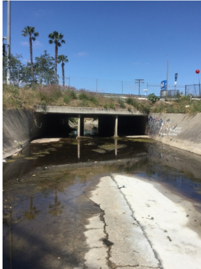
Photo 2: Looking downstream (W) towards 11'x8' triple box culvert underneath Mission Gorge Road in Reach 1
