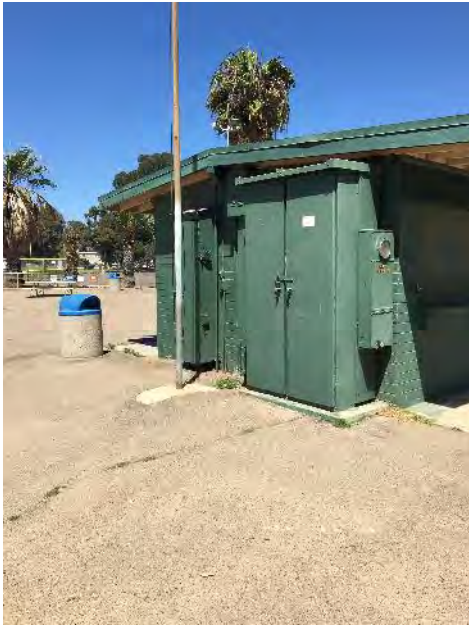
Photograph 52 – Transformer for one of the small buildings associated with the athletic fields. No signs of staining.
