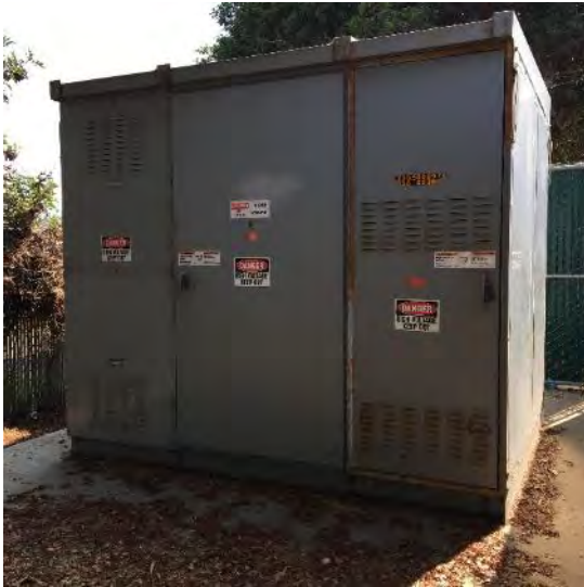
Photograph 76 – The main transformer serving Campland.
