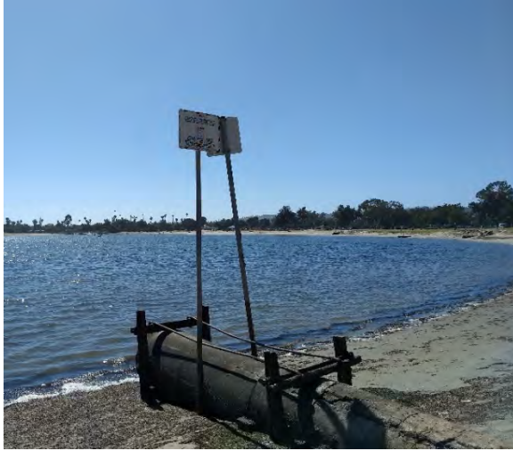
Photograph 5 – One of four storm-water drains along De Anza Cove Park that outlets to Mission Bay.
