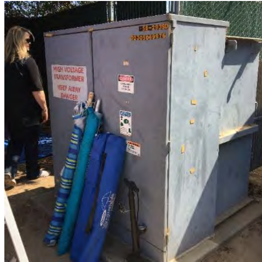
Photograph 77 – One of the smaller transformers. Facilities manager stated that none of the transformers are more than 10 years old.
