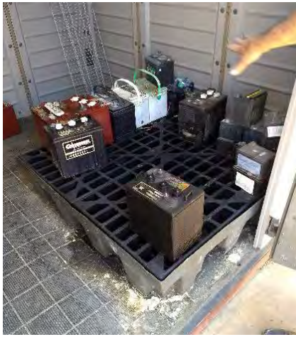
Photograph 80 – A storage shed at Campland contains new and retired batteries. Batteries pictured are no longer in use. Battery acid residue was present beneath secondary containment (on shed floor).
