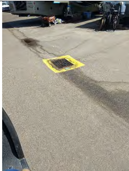
Photograph 67 – Roads through Campland have low area in center with storm drains such as this.
