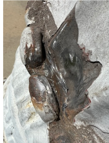
Soldered pole to base joint.
