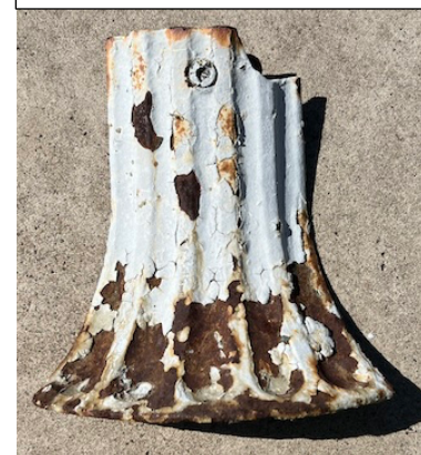
Broken hand hole cover.
