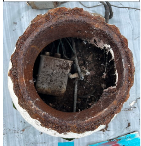
Internal corrosion of cast iron base.
