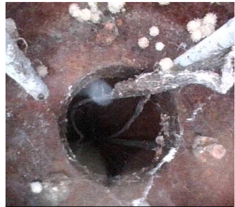
Corrosion of internal assembly rods
