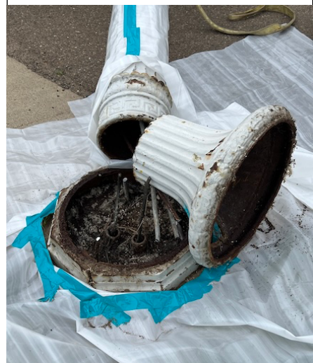
Three sections of the cast iron base.
