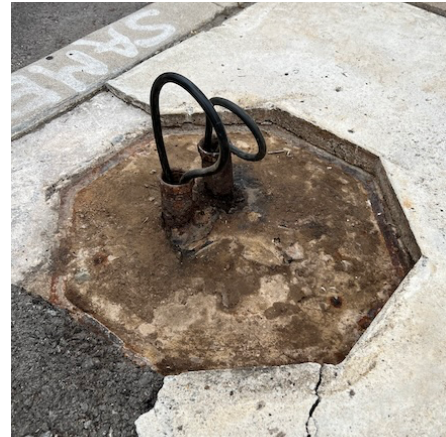
Circuit 2 anchor bolts disintegrated by corrosion over time
