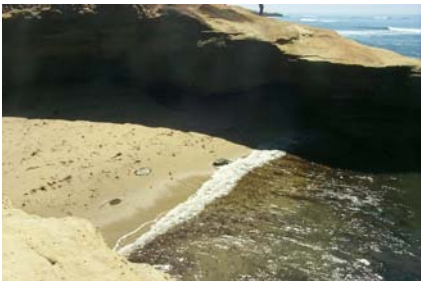
Limit activities to viewing sea caves from distance due to potential safety and ecological concerns. Leave sea caves undisturbed.
