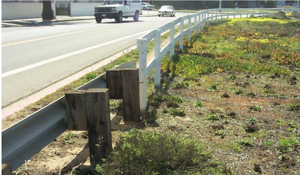
FIGURE 22 - Existing Conditions: Non-compatible barriers and lack of pedestrian access.
