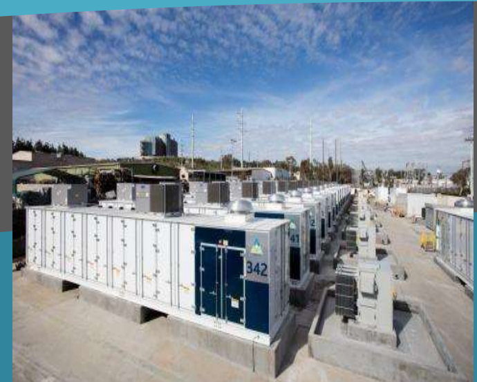
"Expedited Storage Project" Escondido – 30 MW / 120 MWh Array
