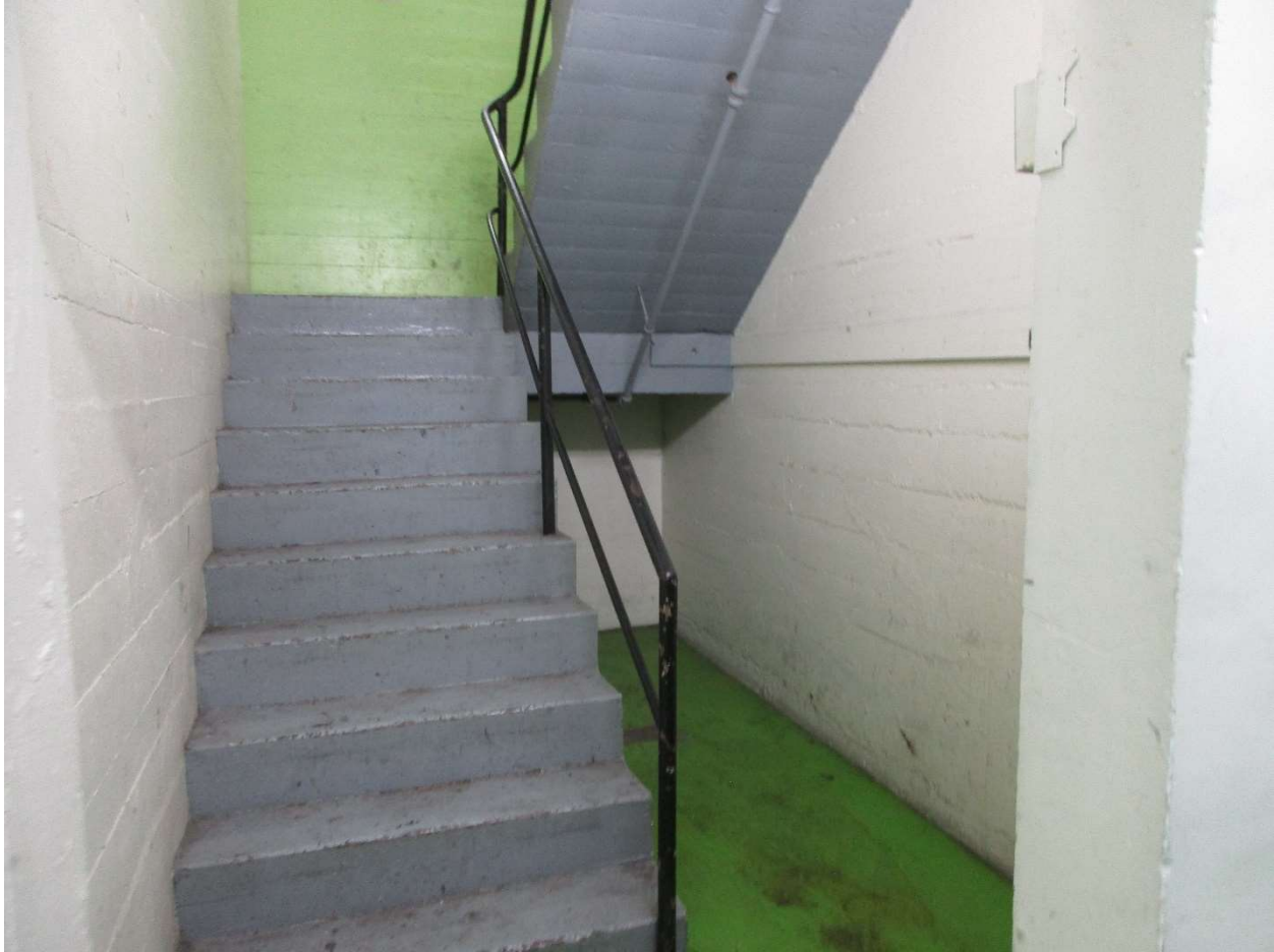
16 CAST-IN-PLACE CONCRETE STAIRS WITH METAL RAILING. STAIR CORE WALLS ARE CONSTRUCTED FROM BOARD-FORMED CONCRETE. LOOKING NORTH IN THE CENTRAL STAIR CORE AT THE FIRST FLOOR.
