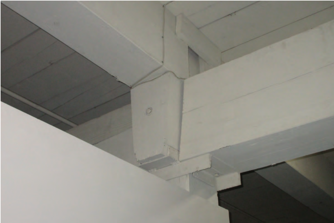
Figure 3-12: Typical wood timber column with steel c-channel capitals field welded back to back supporting the wood timber beams.
