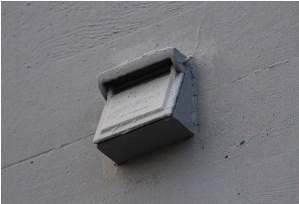
Figure 16: A cast-iron floor scupper with a hinged door. These facade features will be protected-in-place.
