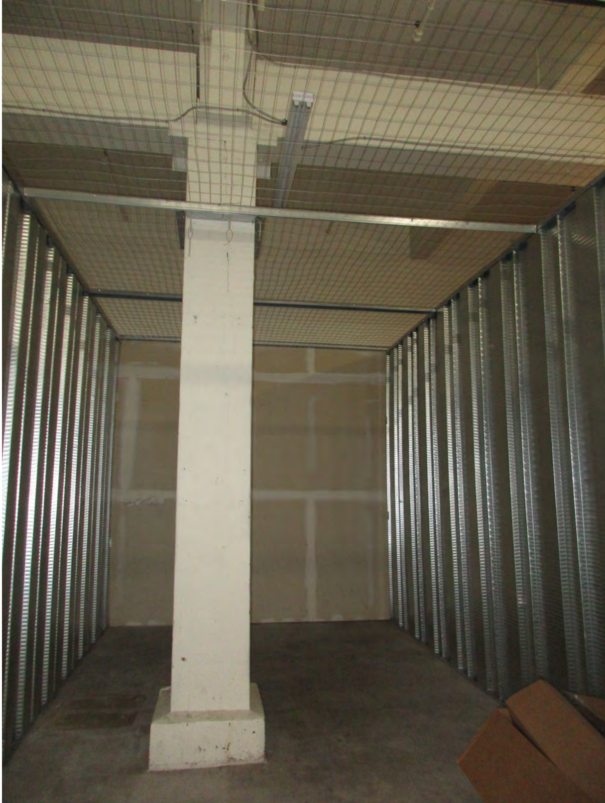
14 LOOKING SOUTH AT THE INTERIOR OF A TYPICAL CORRUGATED STEEL WALL SELF-STORAGE UNIT ON THE FIRST FLOOR.
