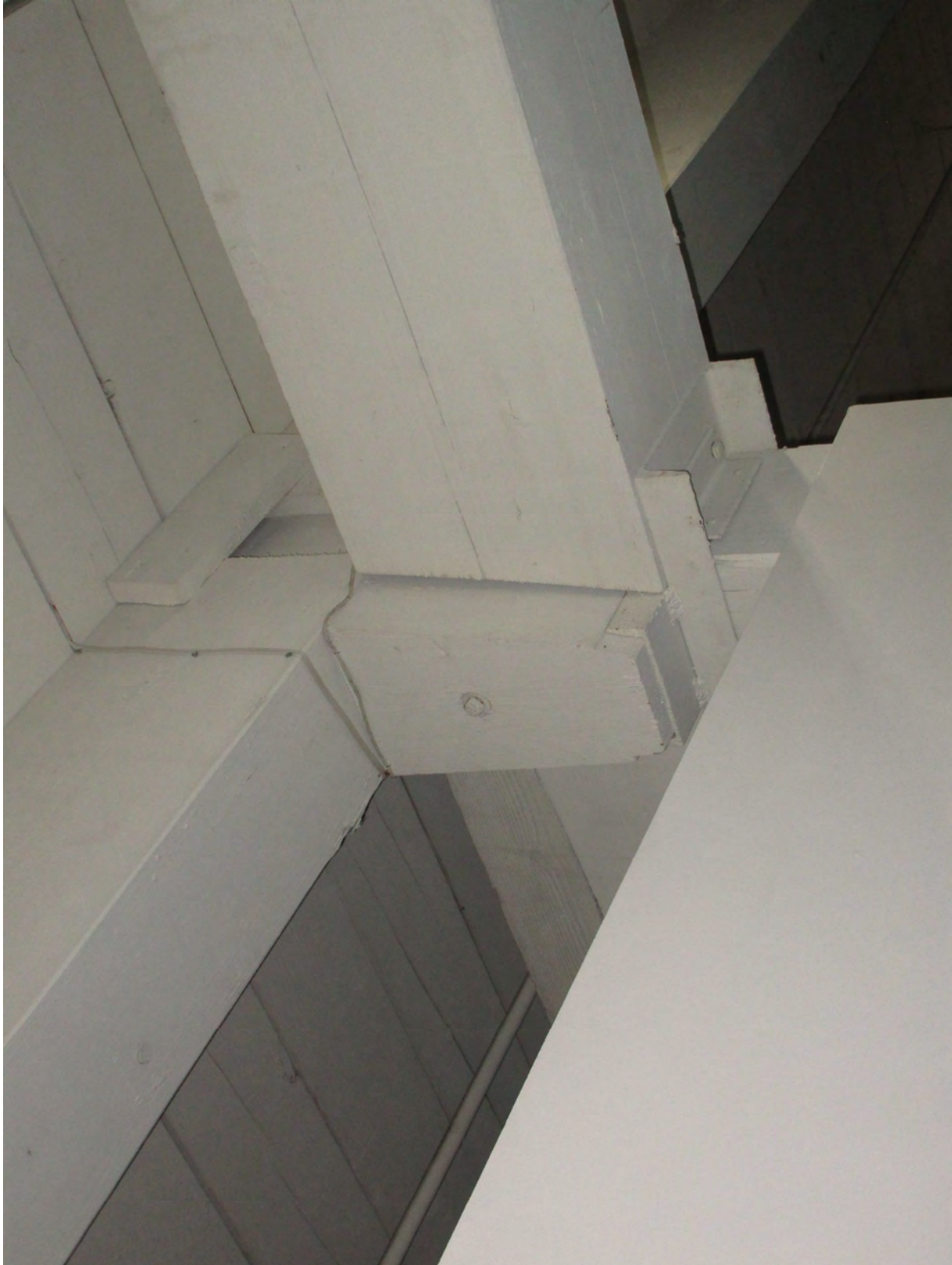
12 TYPICAL WOOD TIMBER COLUMN AND BEAM CONNECTION WITH STEEL CHANNELCAPITALS SUPPORTING THE WOOD TIMBER BEAMS.
