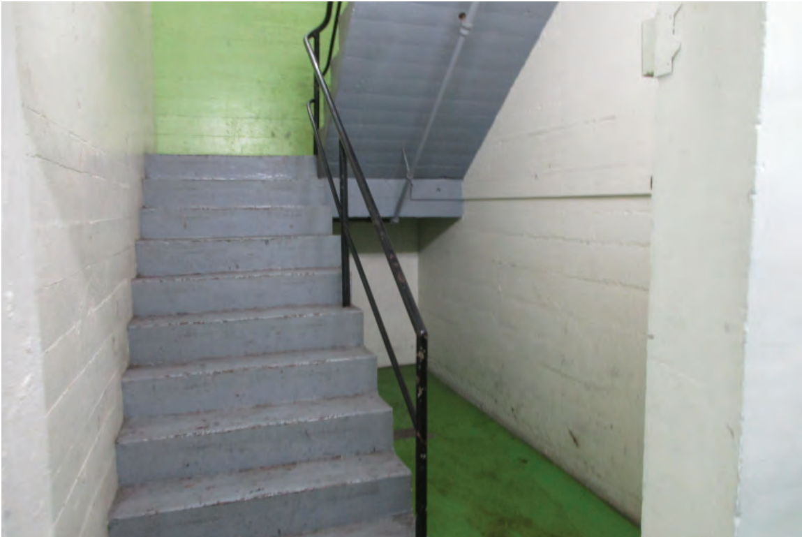
Figure 3-16: First floor, central stair core looking north at the cast-in-place concrete stairs with metal railing. Stair core walls are constructed from board formed cast-in-place concrete.
