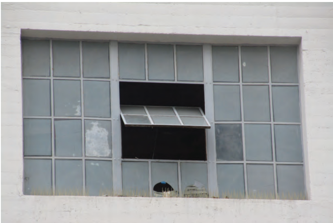
Figure 3-7: A typical historic steel window with a central pivot window and steel mullions.
