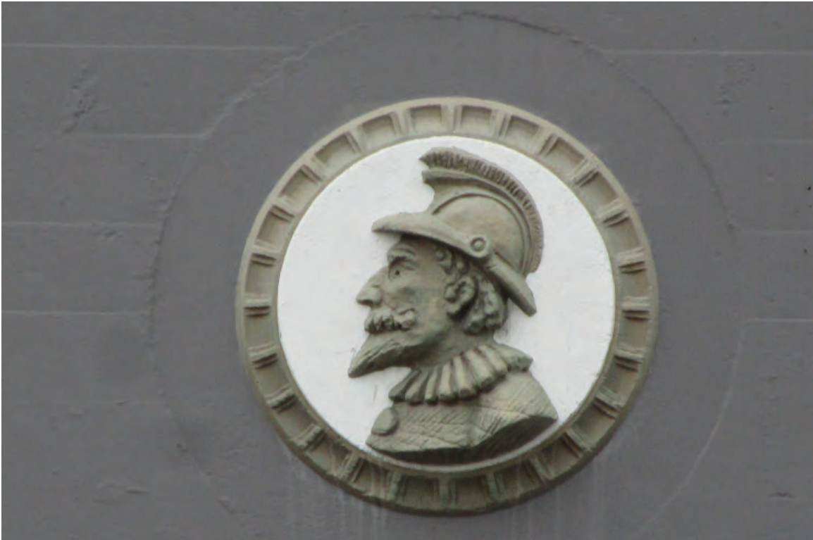
Figure 3-8: Decorative cast-stone shield located above the first floor on the north façade.
