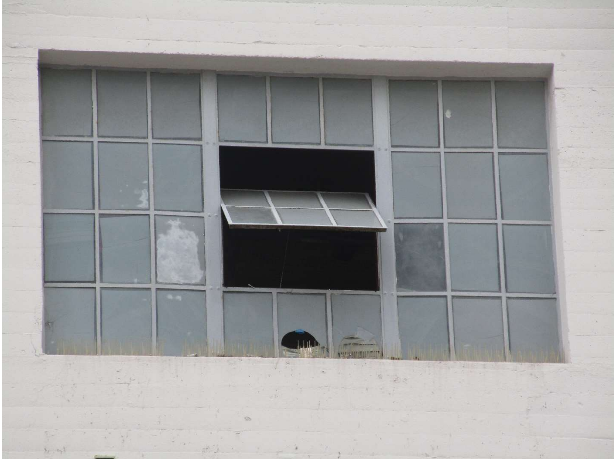
07 A TYPICAL HISTORIC STEEL WINDOW WITH A CENTRAL PIVOT SASH AND STEEL MULLIONS.
