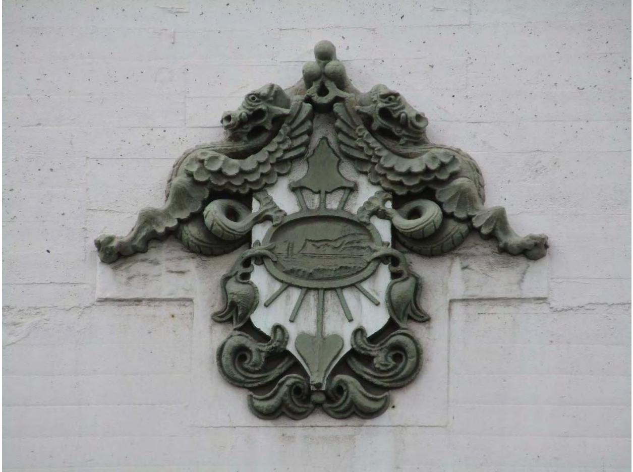
09 CAST-STONE DECORATIVE SHIELD FEATURING POINT LOMA LOCATED ABOVE THE MAIN ENTRY AT THE THIRD FLOOR ON THE NORTH FAÇADE.
