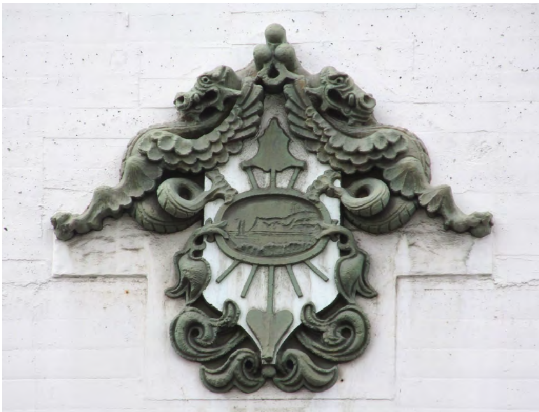
Figure 12: This cast-stone shield features sea monsters and an image of Point Loma. It is on the north facade and will be protected-in-place.
