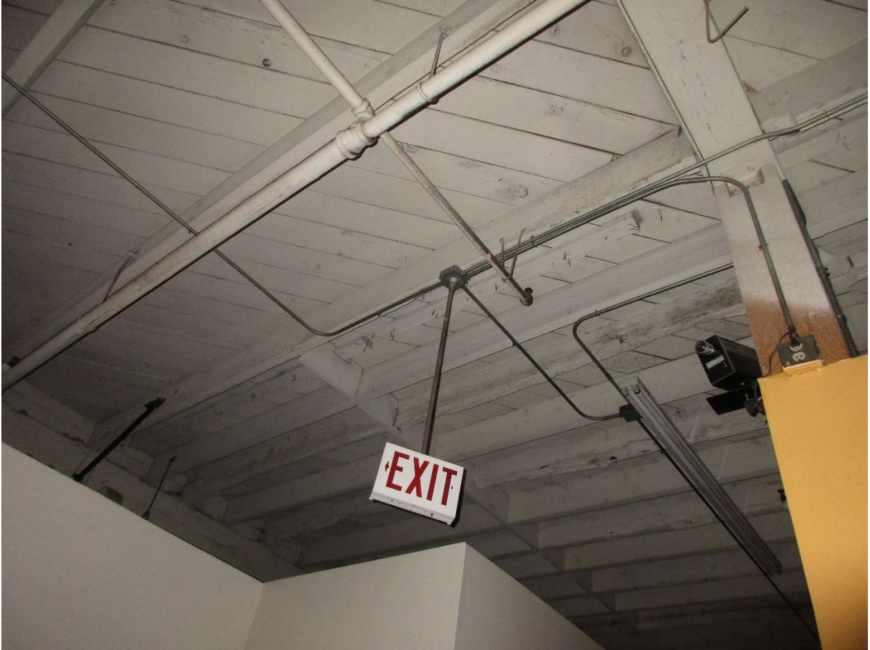
17 LOOKING SOUTHWEST AT THE ROOF FRAMING AT THE WEST WING FORTH FLOOR.
