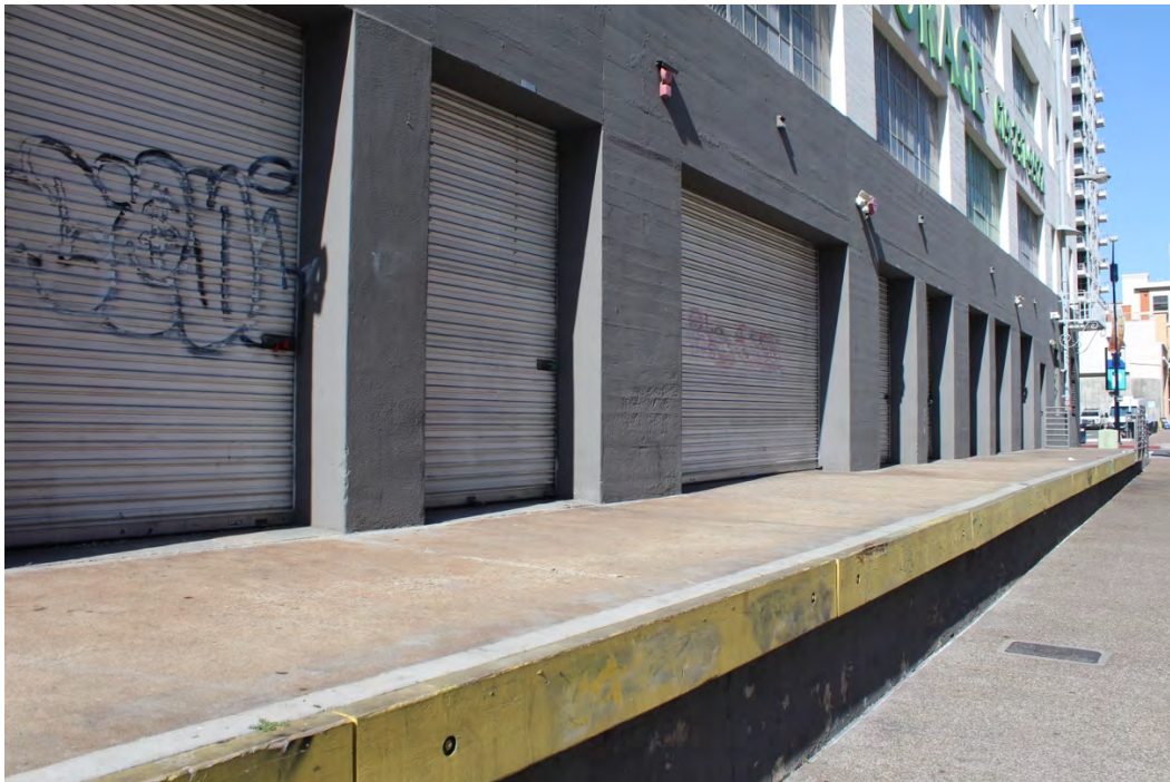
Figure 8: Concrete loading dock and steel roll-up doors on the east side. The dock will be reconstructed with railings and planters added. The doors will be replaced with new glazed storefronts to serve the new uses.
