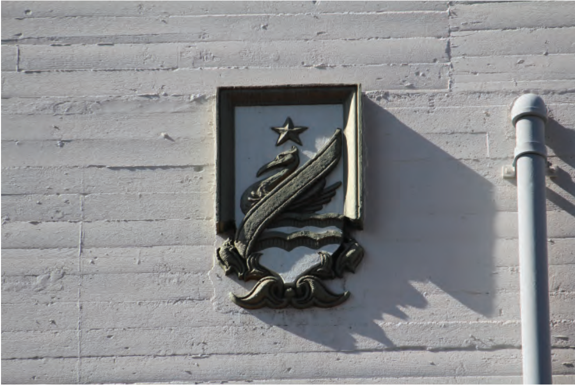
Figure 3-10: Decorative cast-stone shield located at the east end of the north facade. This shield is also used in two locations on the upper east facade.
