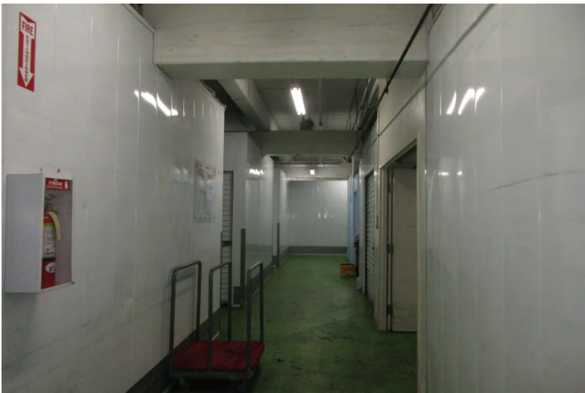
Figure 3-15: Looking south through a typical interior hallway on the first floor. The central elevator core is to the right.
