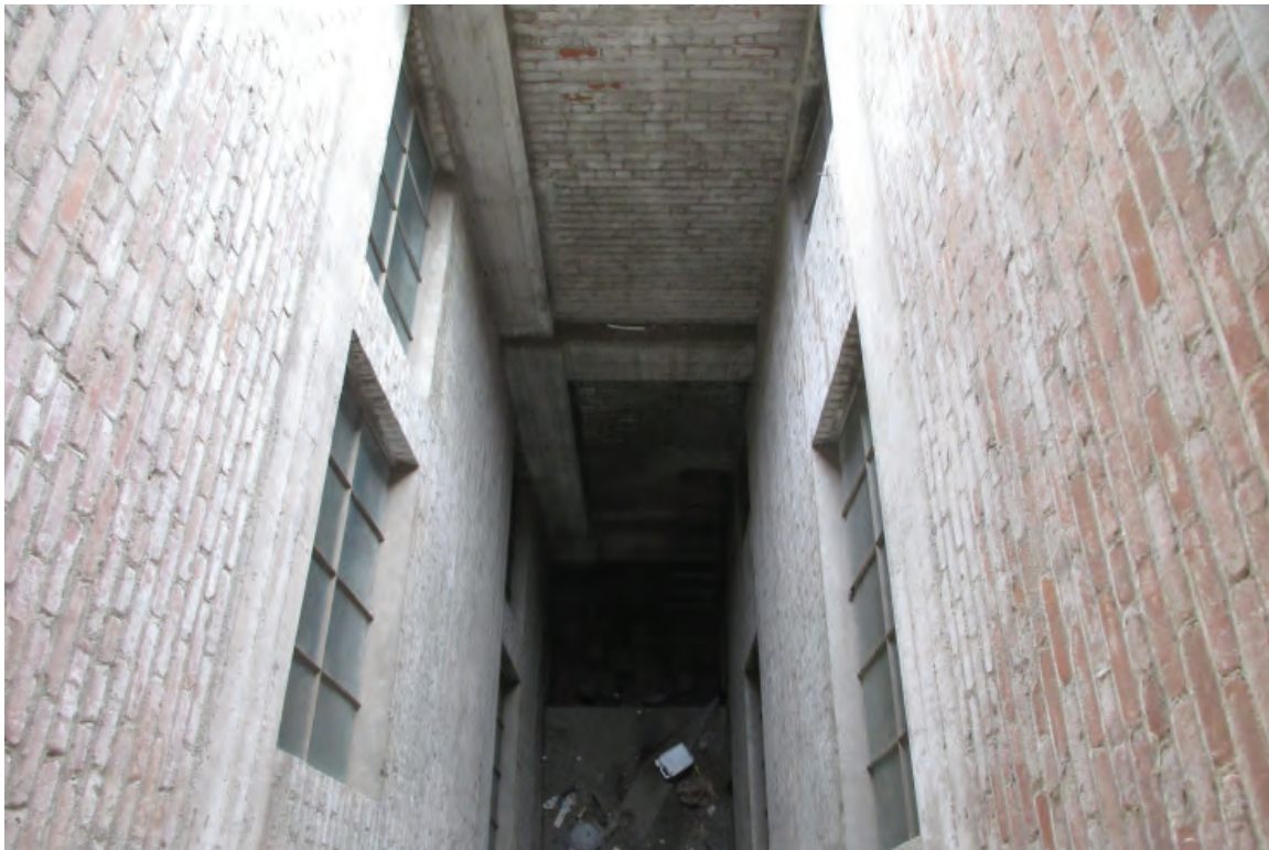
Figure 3-20: The interior of the lightwell at the west side of the east wing.
