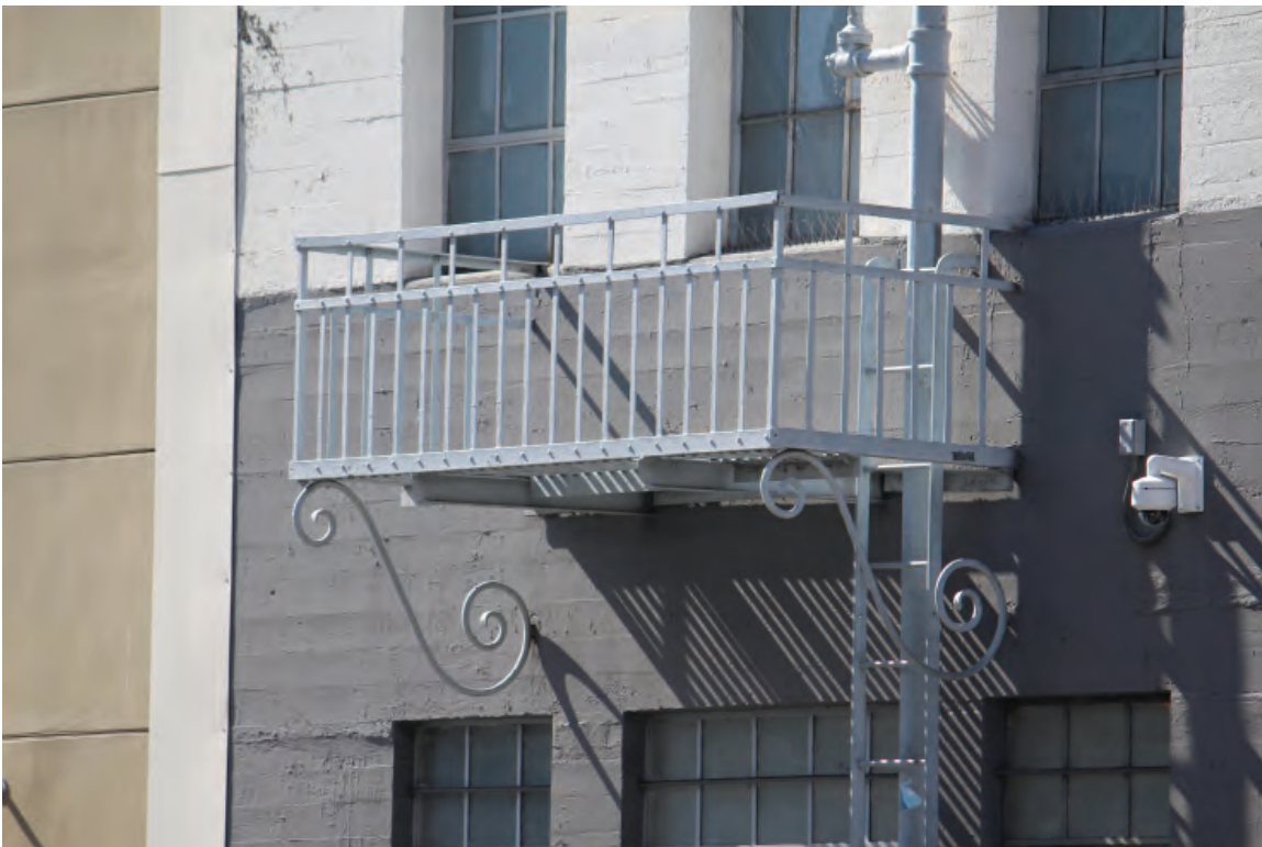
Figure 3-11: Original steel fire-escape balcony at the southern end of the east facade. This shield is also used in two locations on the upper east facade.
