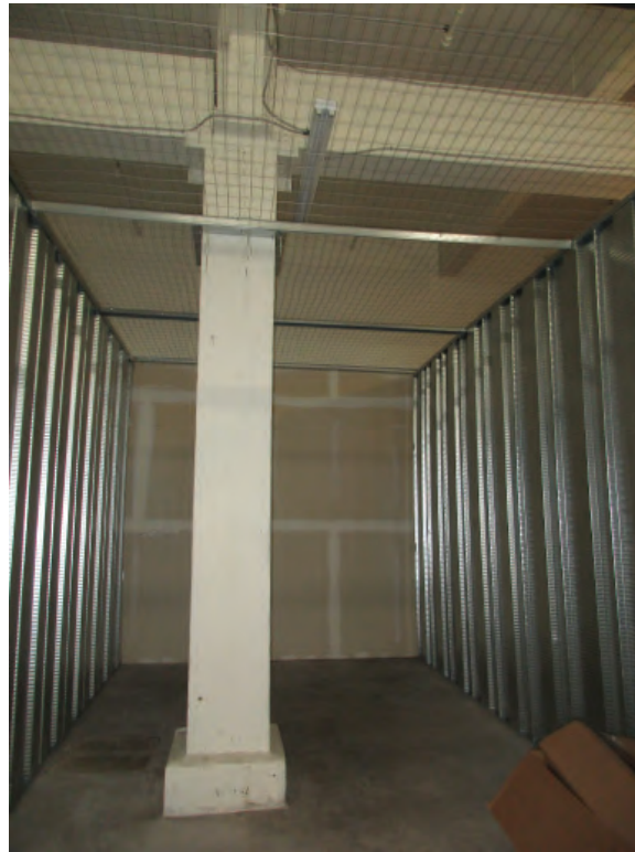
Figure 3-14: Looking south at the interior of a typical corrugated steel wall storage unit on the first floor.
