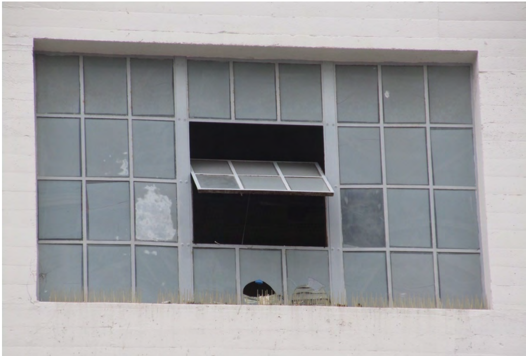
Figure 10: Typical historic steel window with putty-set glazing. Note the added film on the glass. Replace broken and missing glass and restore windows to working condition.
