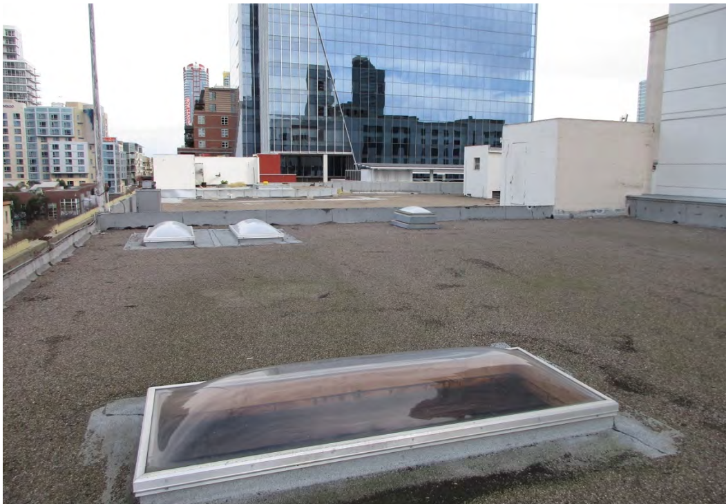
Figure 18: Rooftop view looking east. The roofing, added skylights and penthouses will be removed. The wood flagpole on the left will be retained or replaced in-kind.
