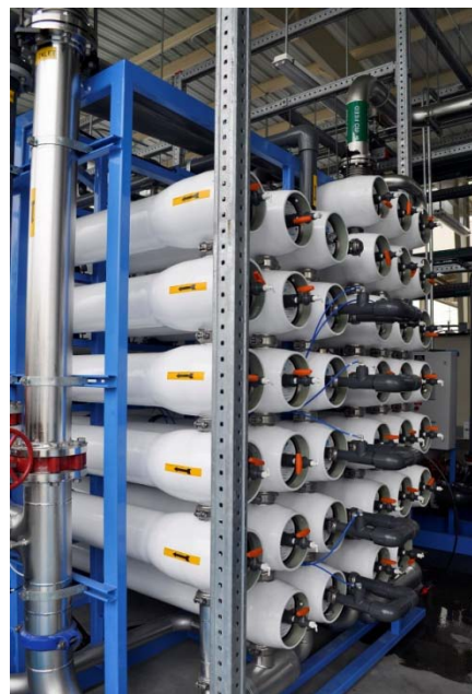
A 15 million gallon day purification facility would be constructed at the City's North City Water Reclamation Plant as part of the first phase of the Pure Water San Diego program.
