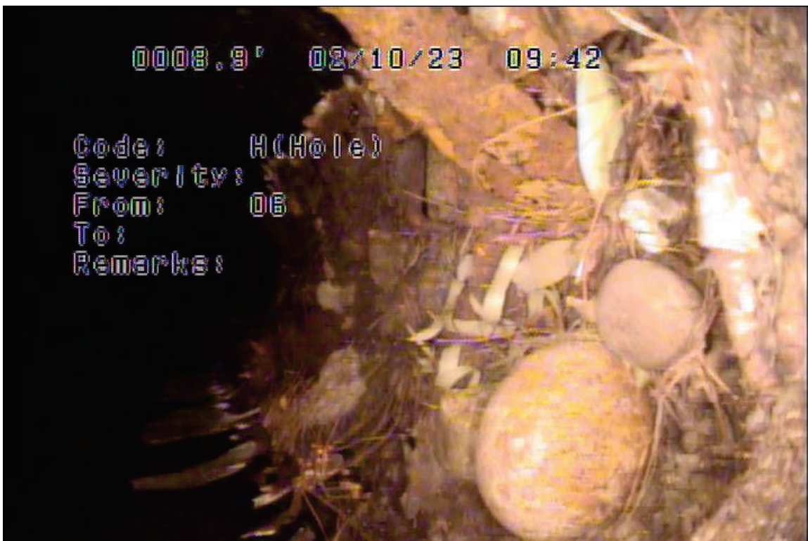
Figure 6 - Bottom of CMP is missing (2/10/23)
