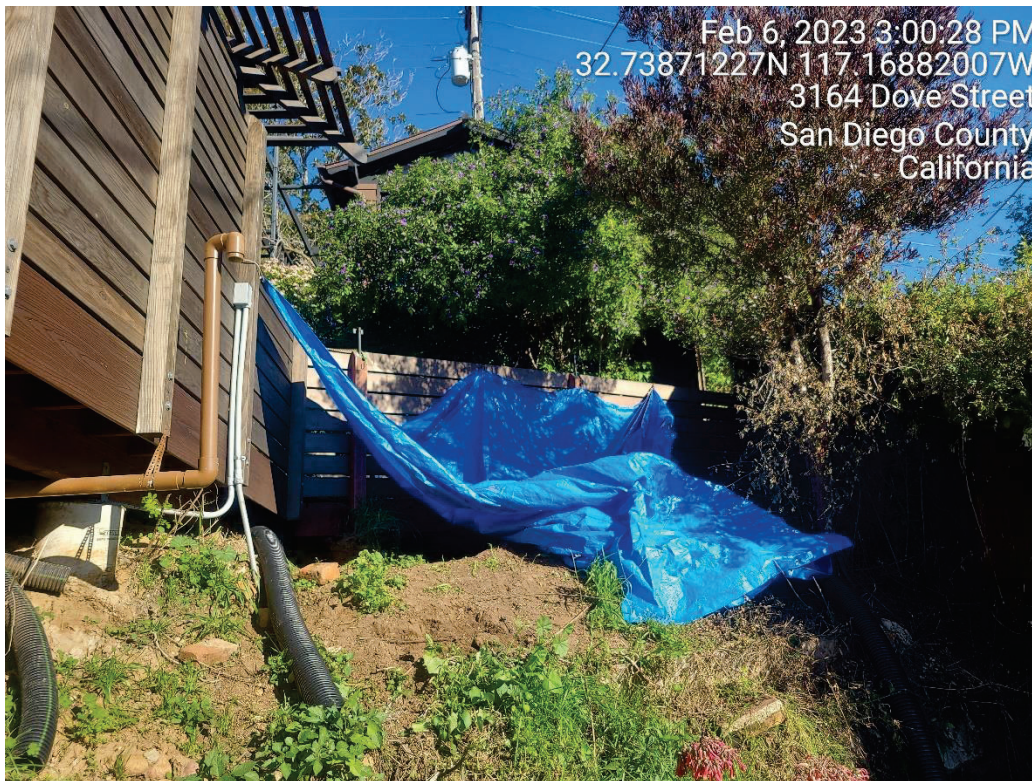
Figure 4 - Sinkhole Vicinity of Adjacent Structures
