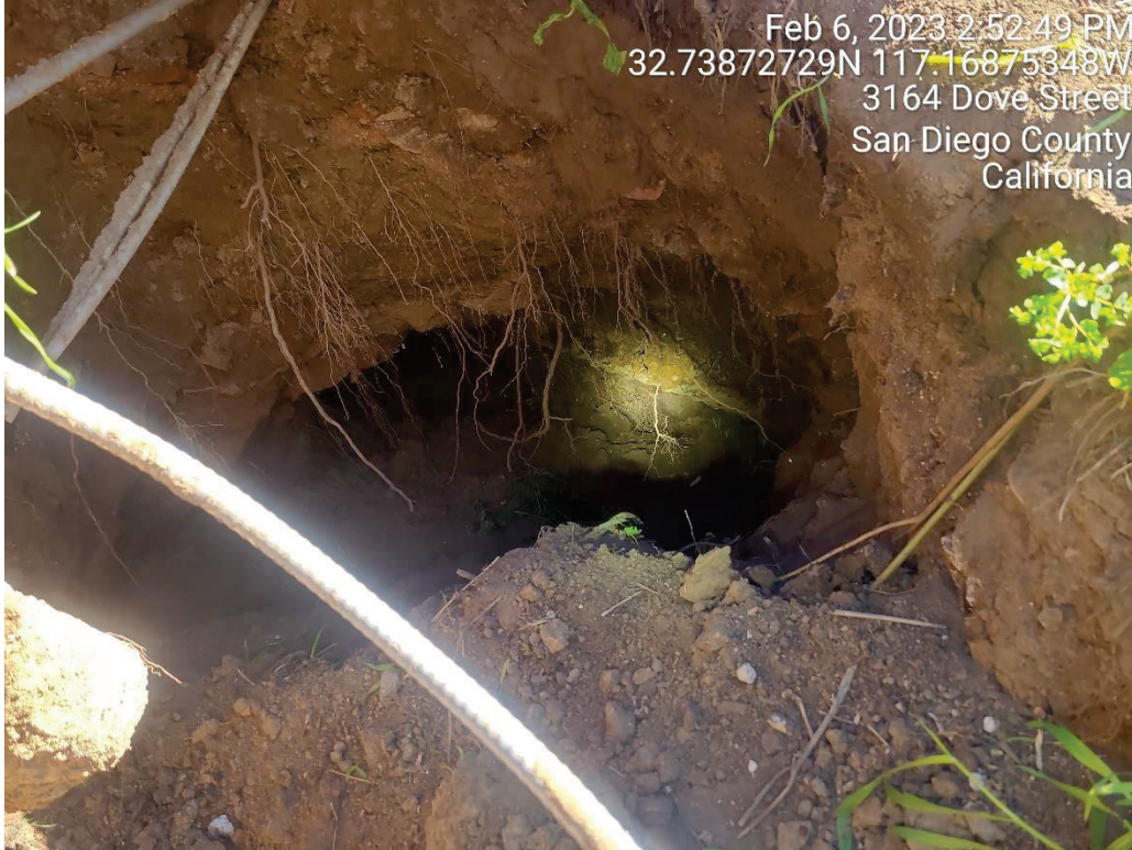
Figure 3 - Exposed Corrugated Metal Pipe (CMP)
