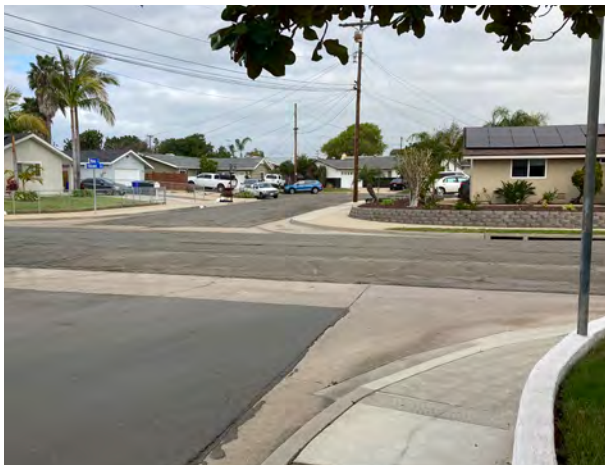
There are several misaligned streets along Hermes Avenue and Hermes Court.
