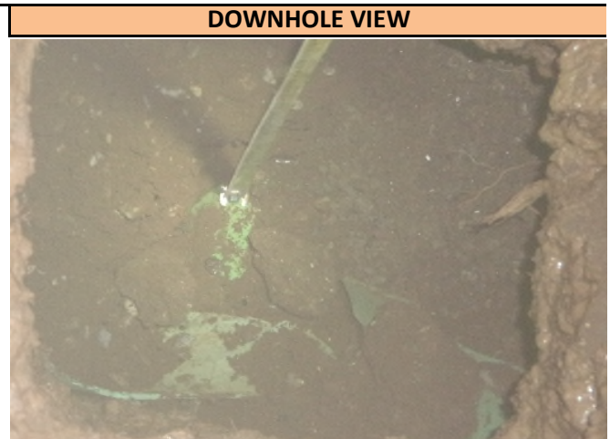
A downhole view of the SDR-35 sanitary sewer utility found in Pothole 3 at the depth of 97 inches T/P. Utility runs in a NW/SE direction at the pothole location and was found directly on markout.
