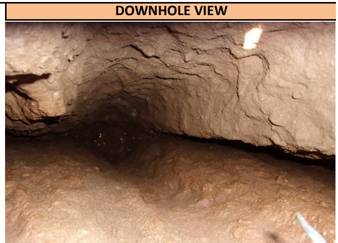
A downhole view of the excavation to 111 inches deep and 36 inches wide. No utilities were found.
