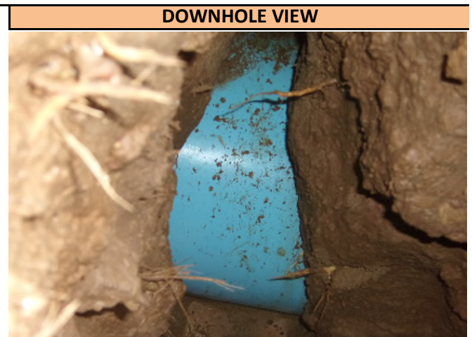
A downhole view of the C900 water utility found in Pothole 1 at the depth of 46.5 inches T/P. Utility runs in a NW/SE direction at the pothole location and was found directly on markout.
