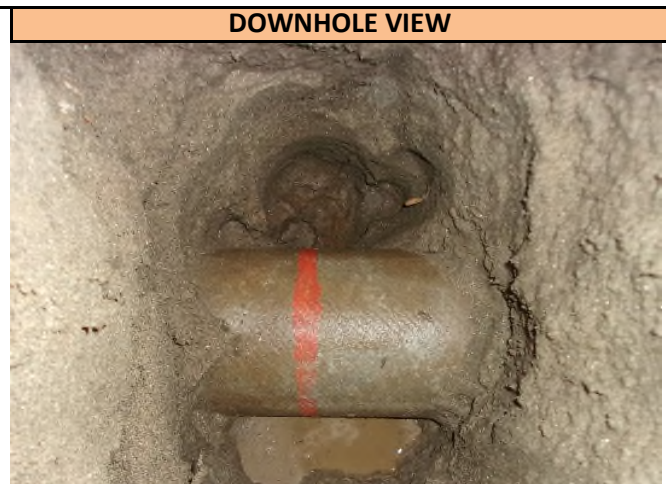
A downhole view of the 6 inch ACP water utility found in Pothole 8 at the depth of 36 inches T/P. Utility runs in a NE/SW direction at the pothole location and was found directly on markout.
