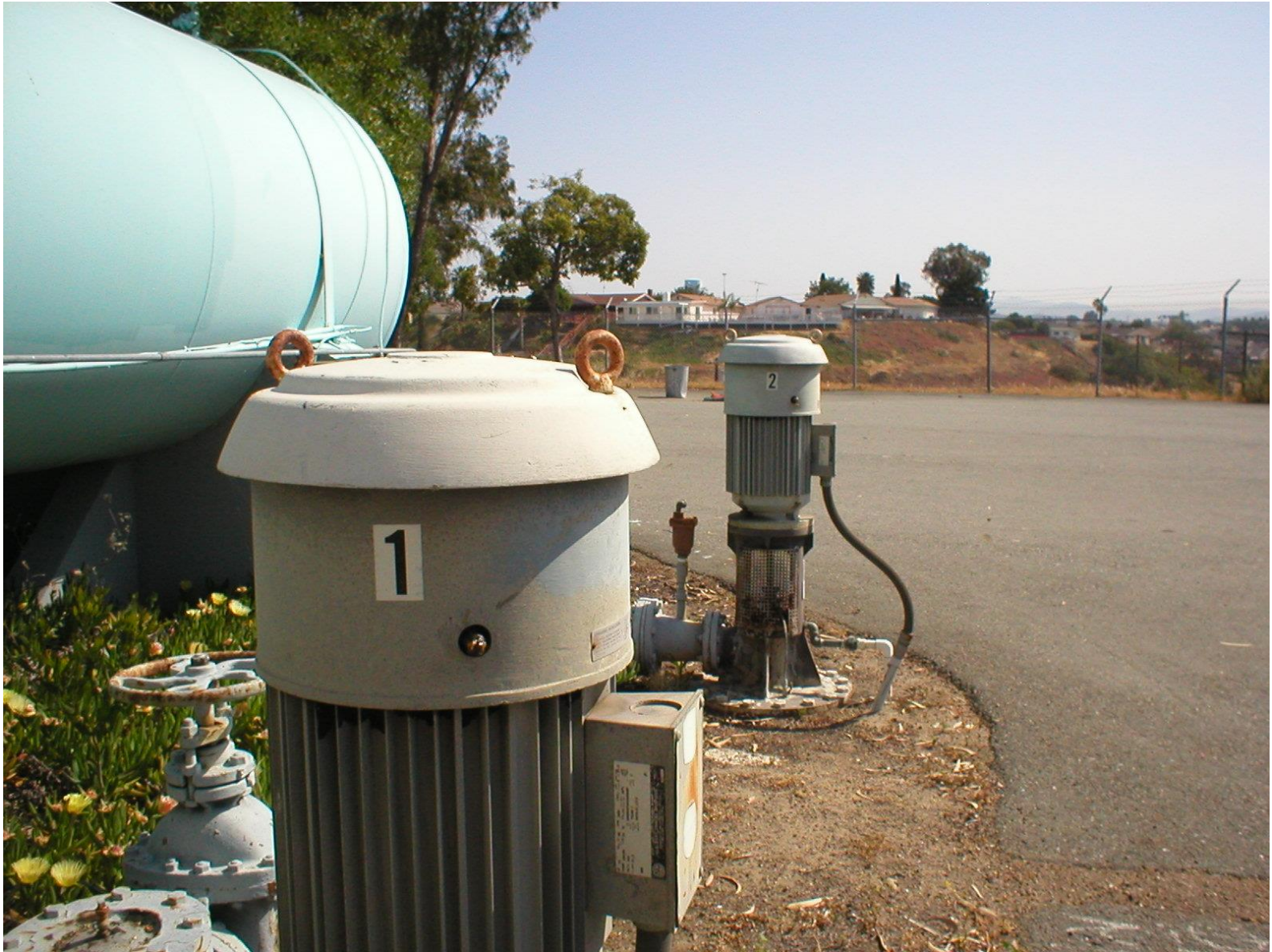
Figure 2. Pump #1 and Pump #2
