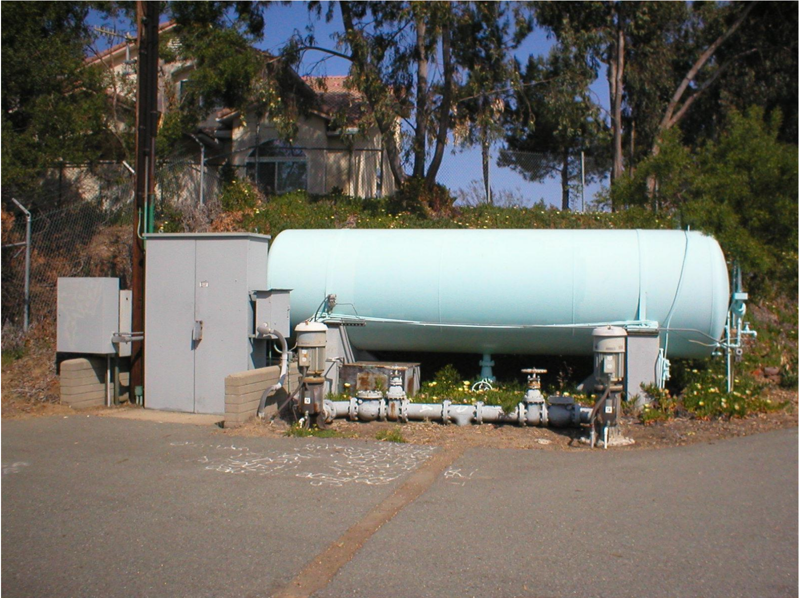
Figure 1 Water Pump Station
