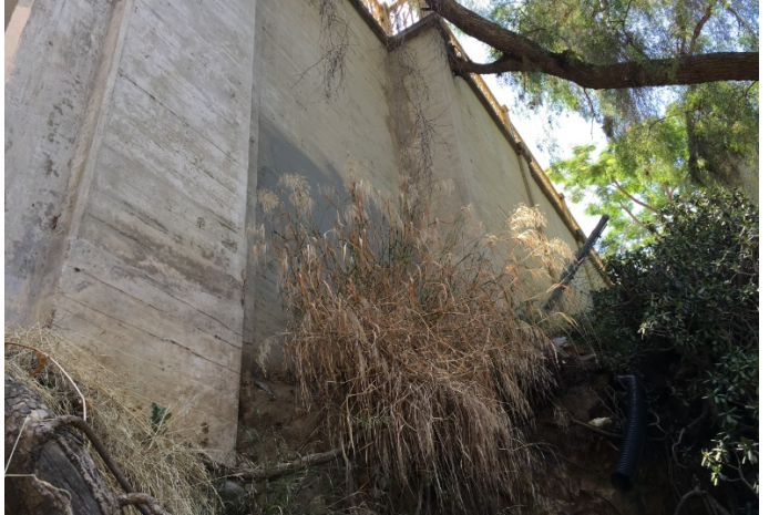
TAKEN FROM THE SINKHOLE LOOKING SOUTHEAST
