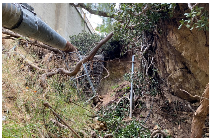
TAKEN FROM THE SINKHOLE LOOKING SOUTHEAST
