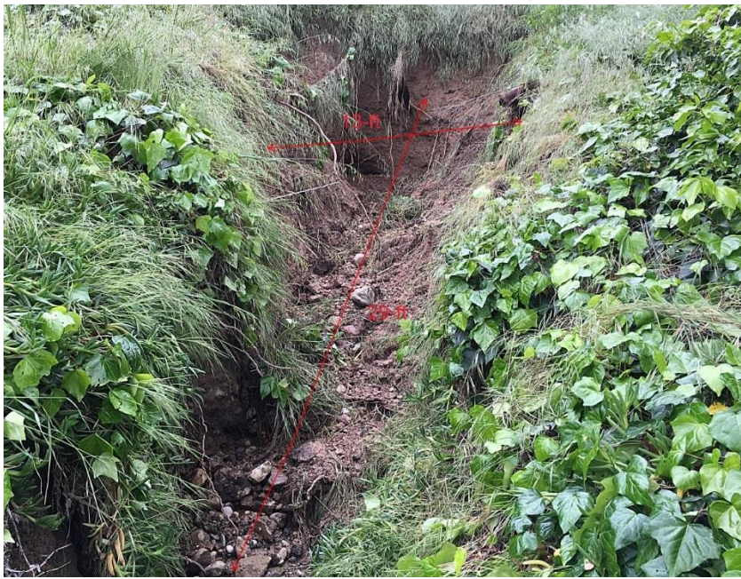
New Slope Failure. Photo taken looking up the slope.
