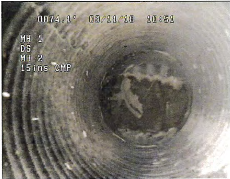
Photo 7 – pipe blocked by debris at about 74 feet from upstream inlet. Looking west.
