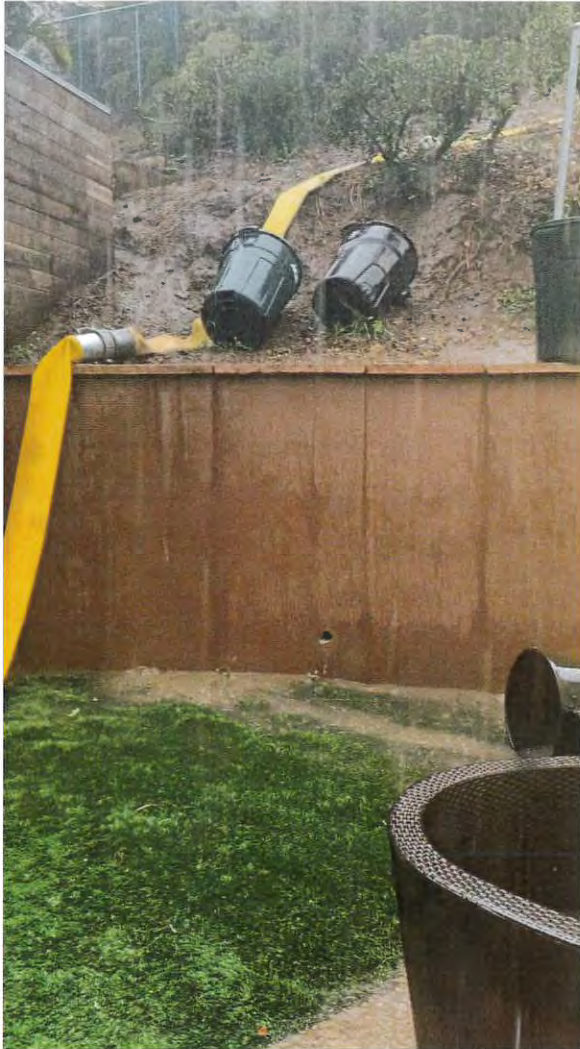
Photo 9 – water bubbling and coming in from underneath the retaining wall.
