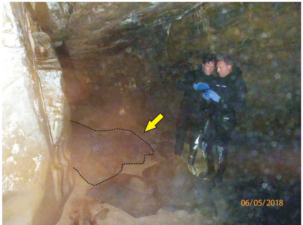
PHOTO 5A: NOTE APPARENT RECENT ROCK DEBRIS (ARROW).
