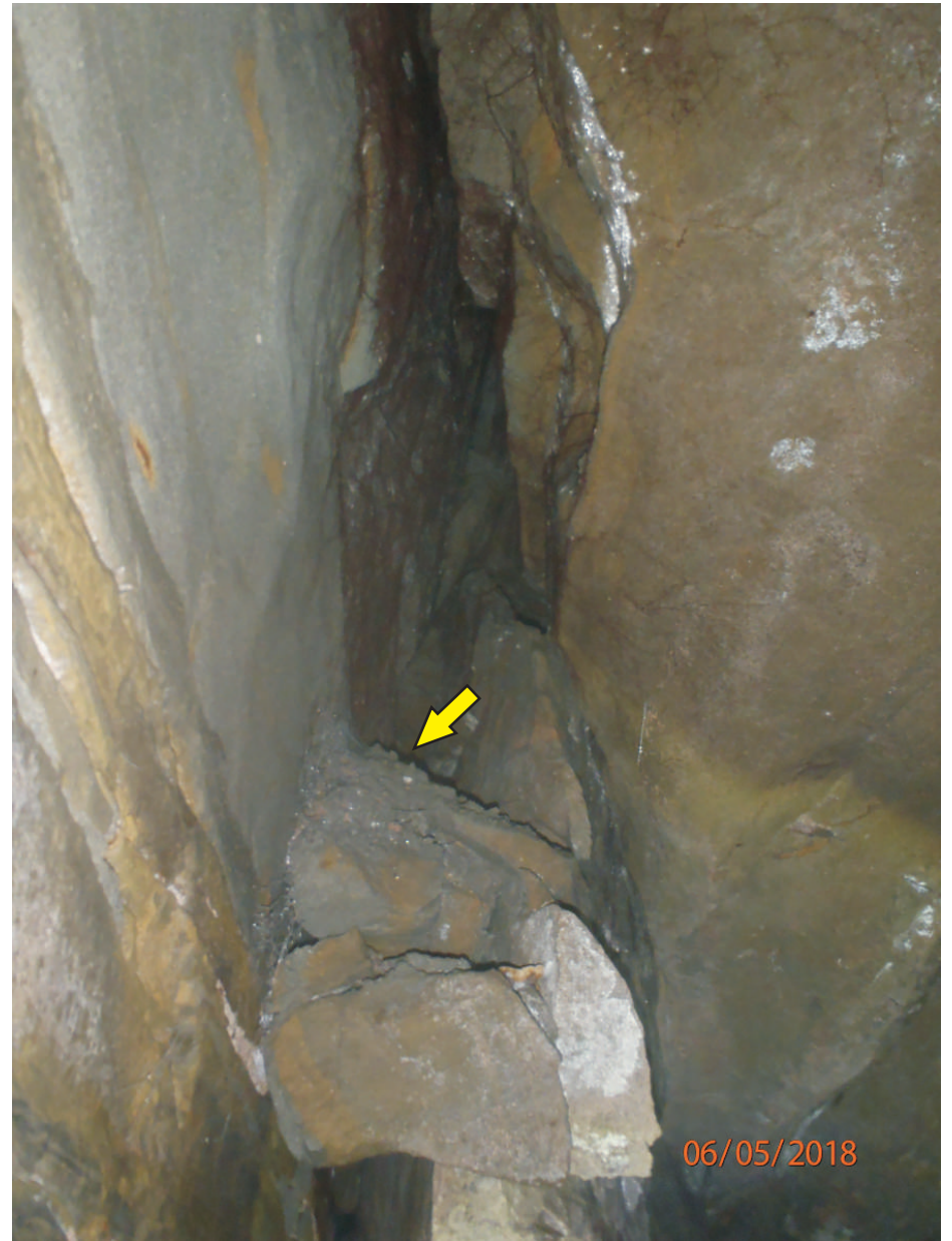
PHOTO 6A: NOTE SAND PIPING FROM OVERLYING TERRACE DEPOSITS (ARROW).
