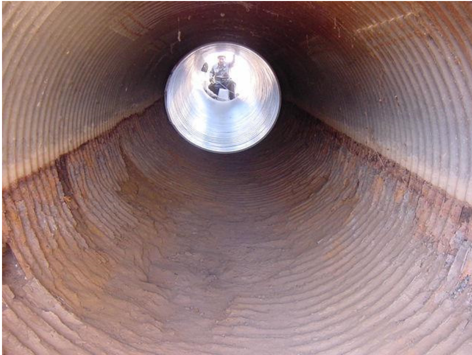
Figure 6: Heavily corroded corrugated steel culvert
