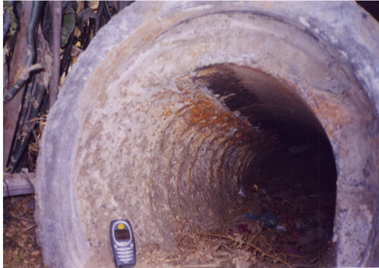
Figure 5: Sulfide-corroded concrete pipe
