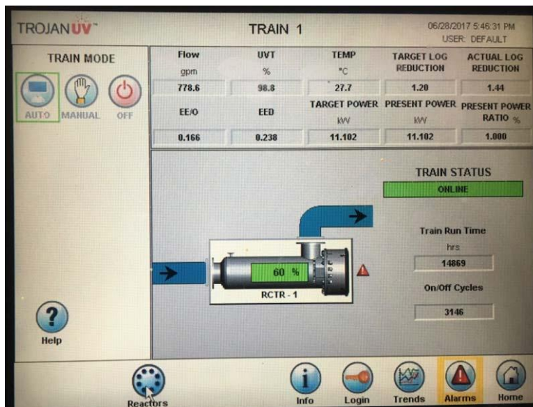
Figure 81. UV/AOP System Train Screen
