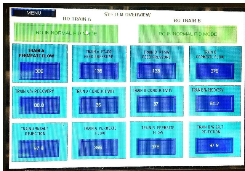
Figure 57. RO HMI System Overview Screen
