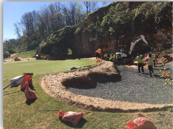
Capillary concrete installation on greenside bunkers with minimal disturbance to existing greens.
