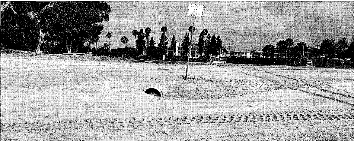
Photograph 14. View of the storm drain outlet on the high beach that is responsible for the majority of the beach shoal development at the northern end of Crown Point Shores. (08-09-16).
