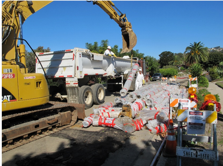
Orion crews removing and disposing AC pipe with proper personal protective equipment (PPE)
