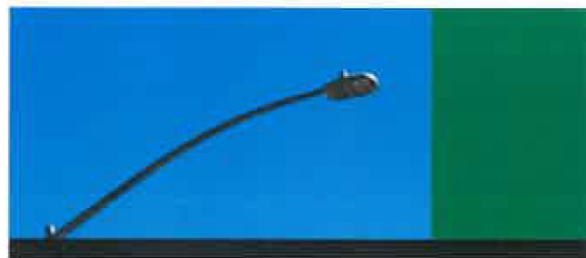
Figure 2: Fairmount Ave Street Lights with GE LightGrid Wireless Node
