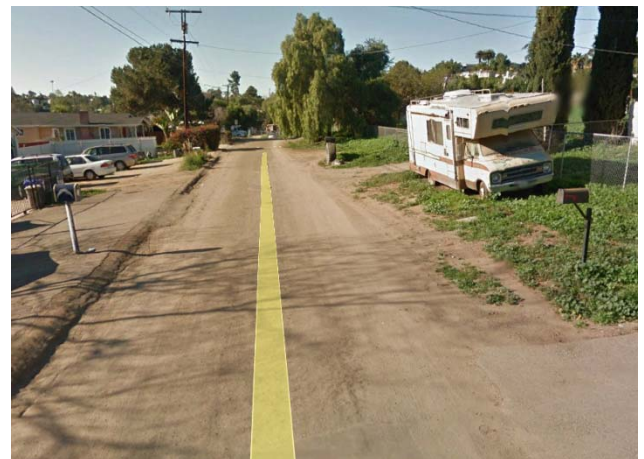
Substandard Pavement on Tarbox St.
