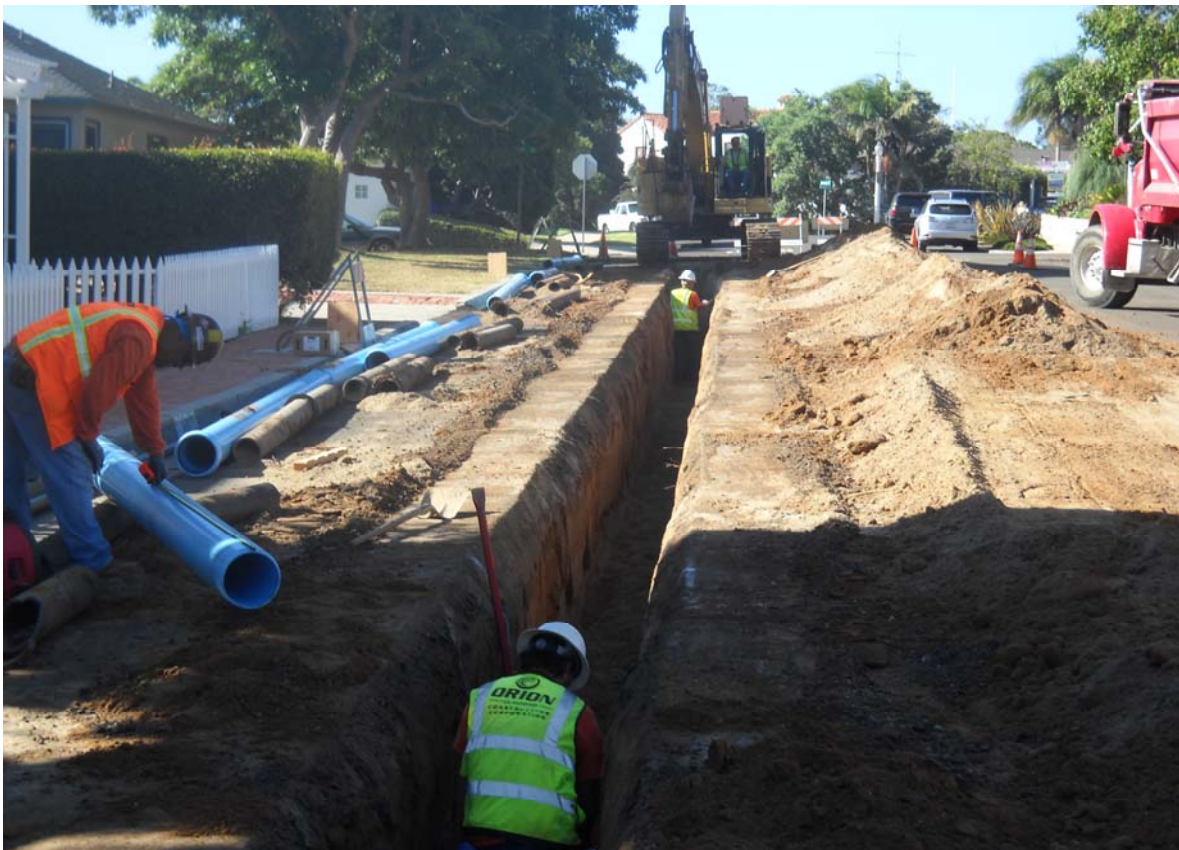
Mainline installation with AC pipe removal integral to the process – the existing AC pipeline is removed as the new PVC pipeline is installed directly back in its place.
