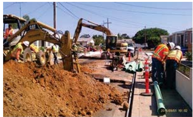
Installation of deep sewer mains, with water highlined in advance. Onsite TCDB huddle with City staff handling unknown utility conflicts while work is in progress.
