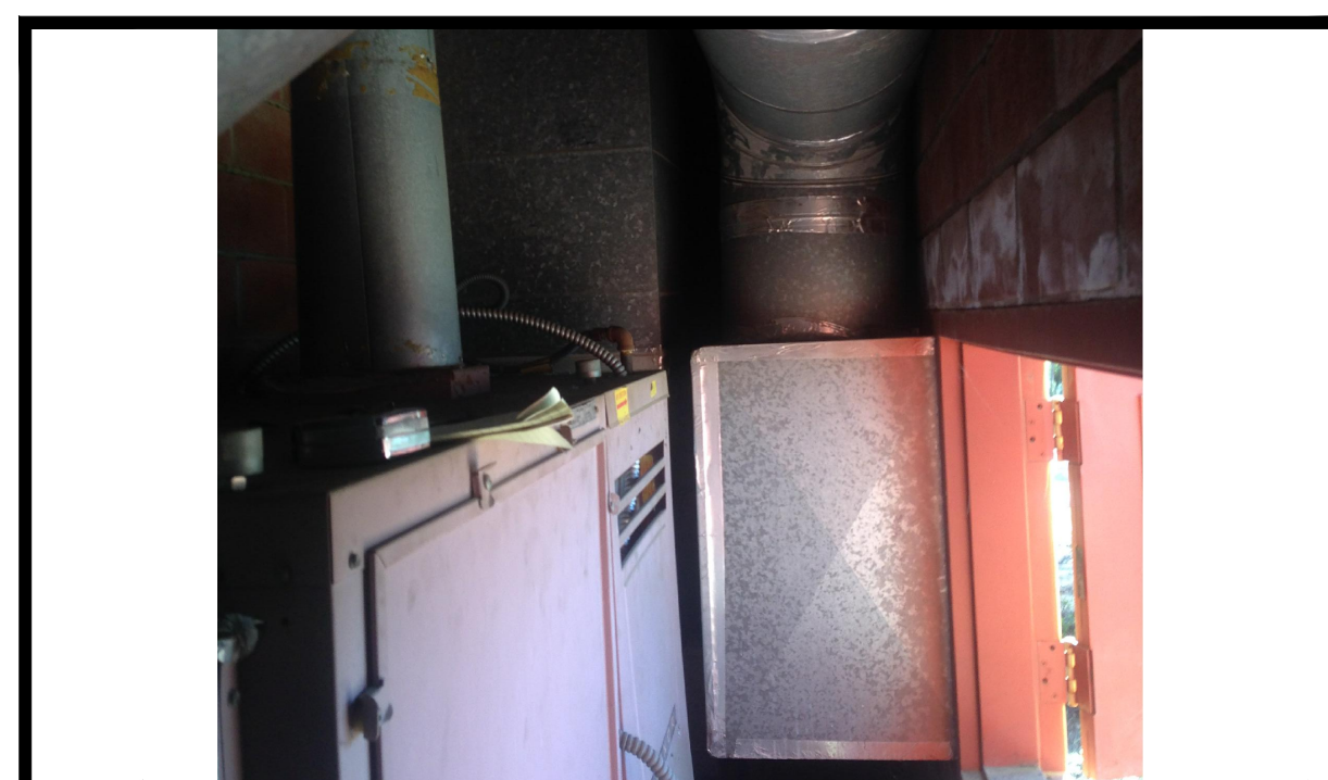
16 MAKE-UP AIR UNIT, MAU-2 TO BE REPLACED.
