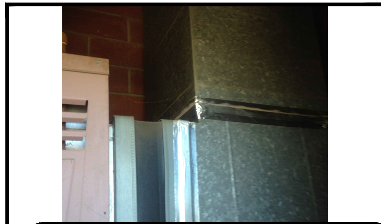
14 MAKE-UP AIR UNIT MAU-1 TO BE REPLACED.
