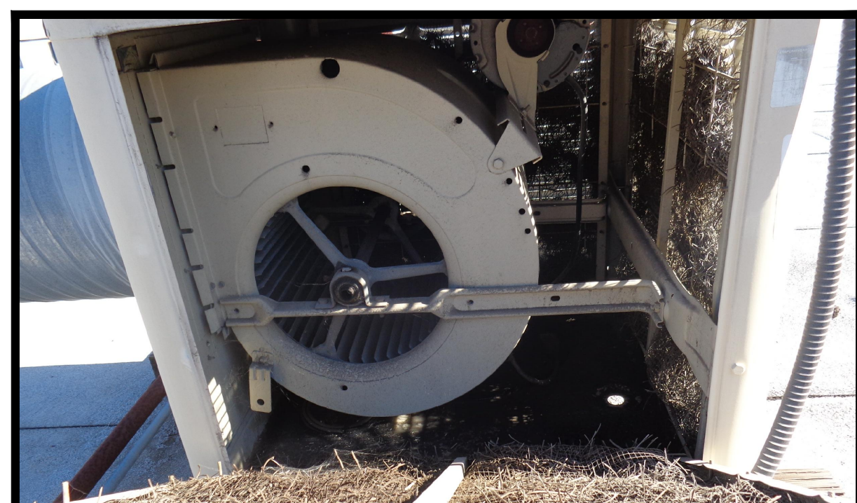
8 SWAMP COOLER TO BE REPLACED WITH SUPPLY FAN.
