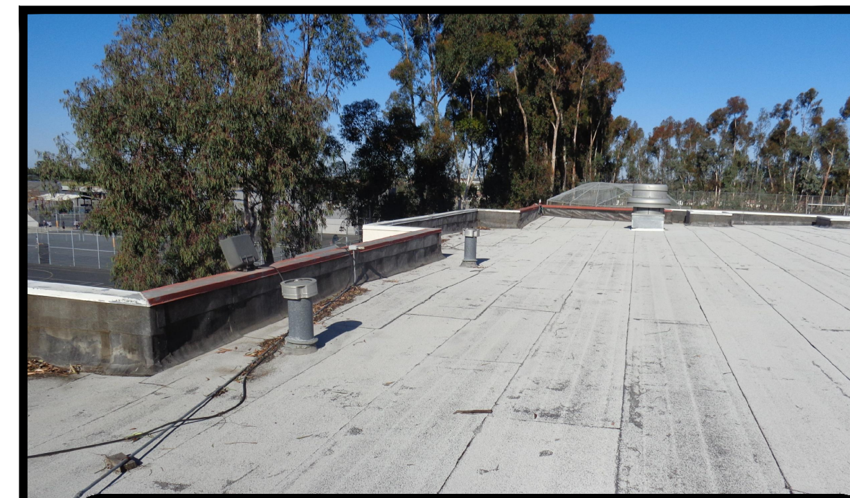
2 VENT FROM MAKE UP AIR UNIT, MAU-1 AND MAU-2 TO BE REPLACED.
