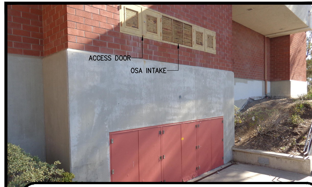
13 ACCESS DOOR FOR MAKE-UP AIR UNITS.
