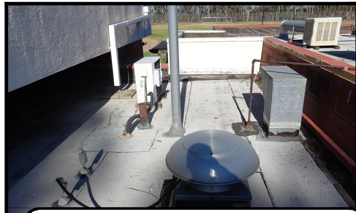
5 EXHAUST FAN EF-6 AND CONDENSING UNIT.
