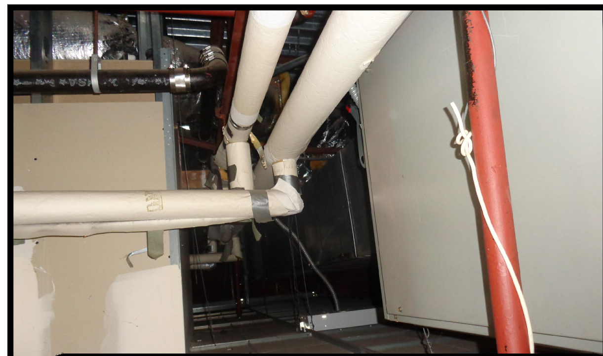
11 AIR HANDLING UNIT AH-1 TO BE REPLACED.
