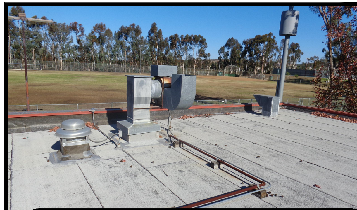
10 EXHAUST FAN EF-7 AND EF-9 TO BE REPLACED.
