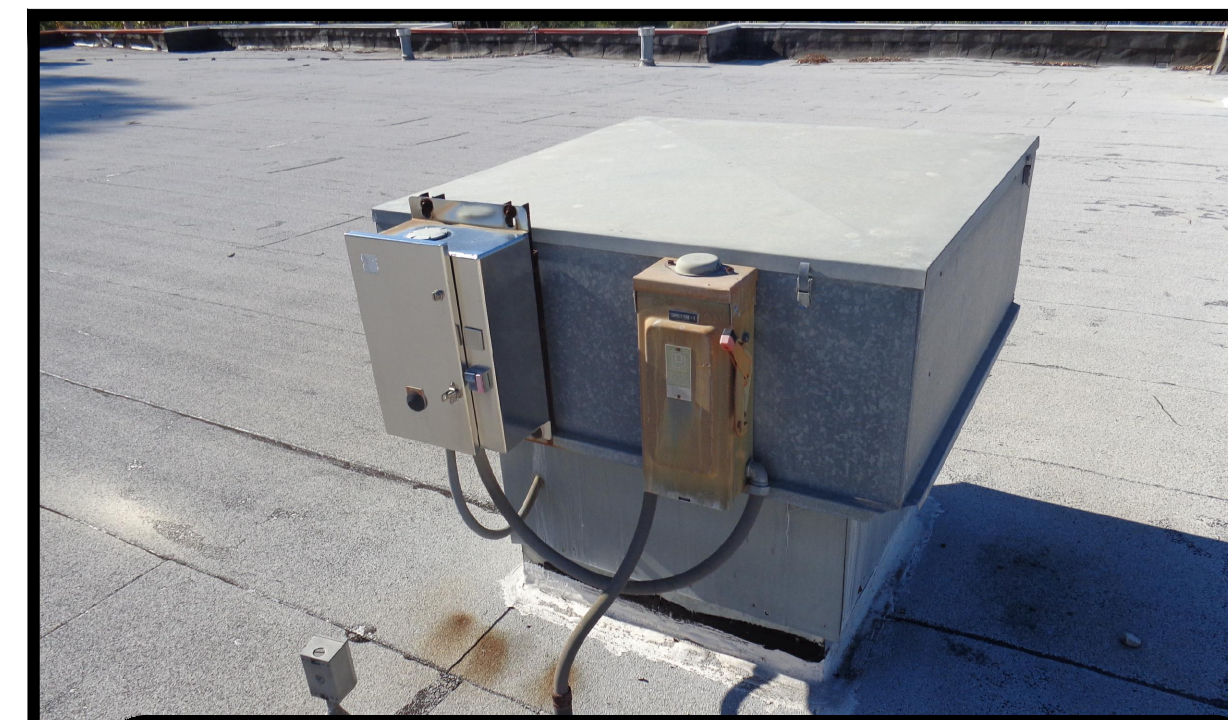
3 TYPICAL SUPPLY FAN SERVING GYM TO BE REPLACED.
