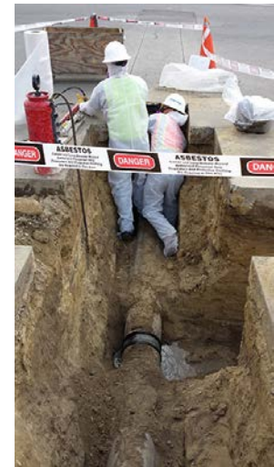
Proper asbestos pipe removal and disposal by a Casper Company for TC on MACC 1, Task Order 1, Skyline Avenue in front of Morse High School.
