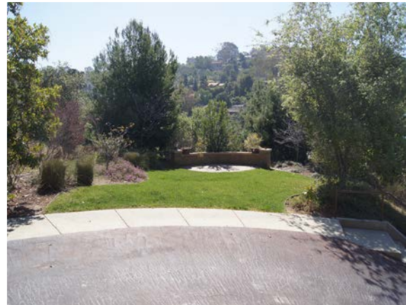
Driveway at the end of the cul-de-sac on Fairway Road, HDD jacking pit will be located here.
