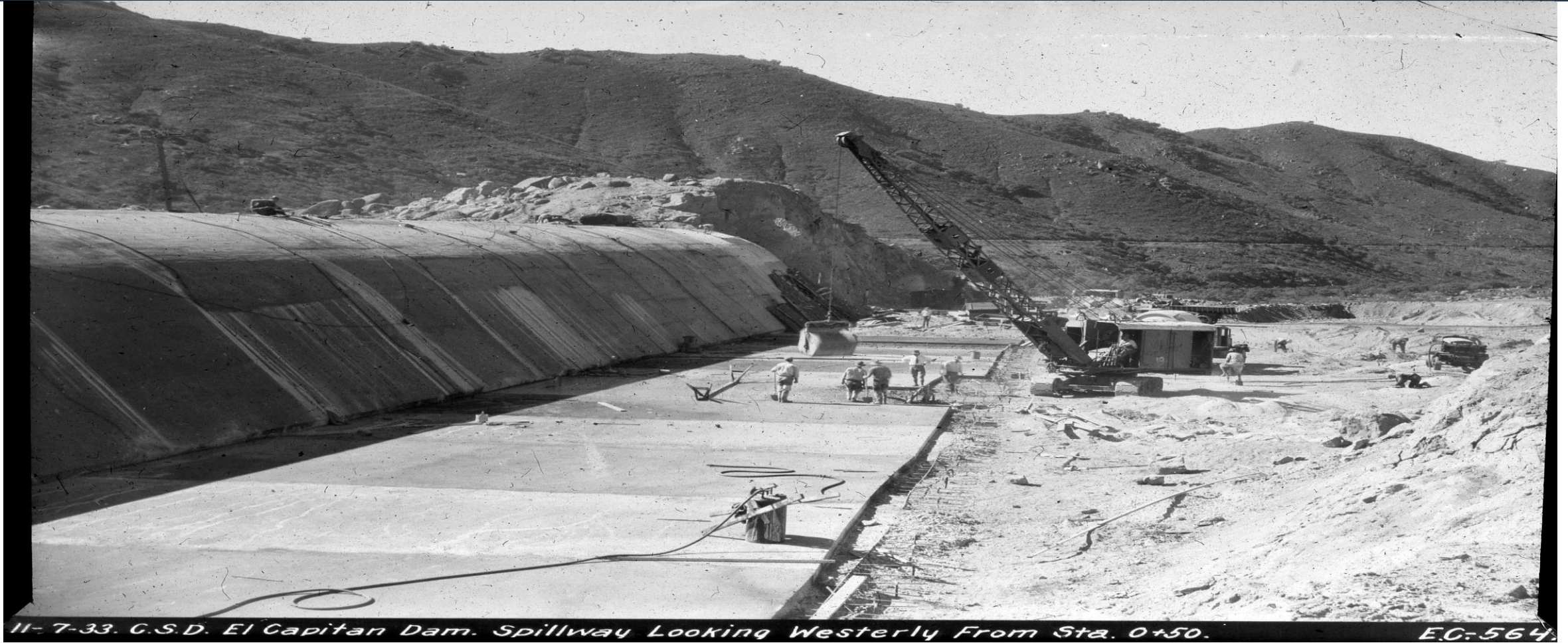
City of San Diego El Capitan Dam – Laying the Foundation while Looking West 1933
