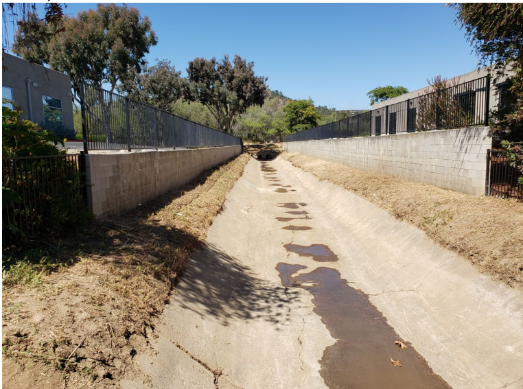
Flintkote post maintenance photo looking near Roselle Street east towards culverts that enter the Roselle channel (June 25, 2022)
