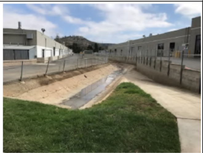
Flintkote Post-Maintenance - Photo 1: view of Flintkote 1 looking northeast. Taken from western edge of project site. Maintenance activities shown to be complete (November 4, 2021)
