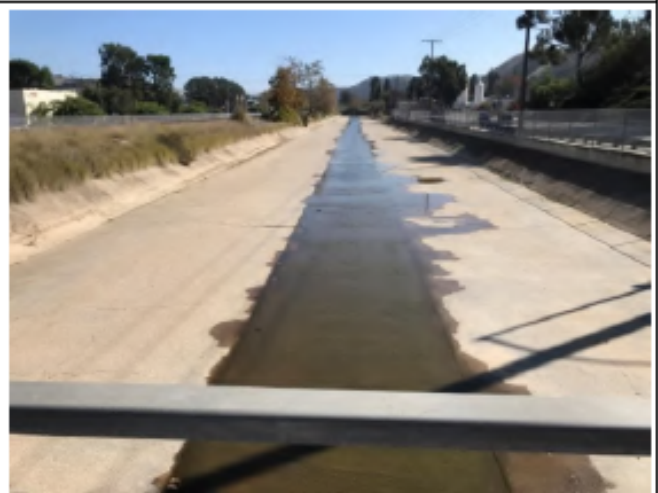
Roselle Post-Maintenance - Photo 11: view of Roselle 2 looking east from approximately the center of the channel showing vegetated and unvegetated sections of concrete-lining.
