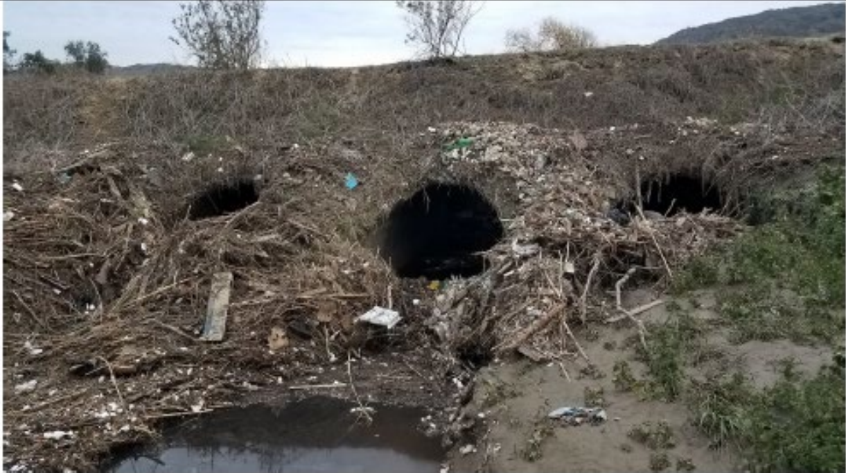
Photo 2: Pre-construction photo showing trash and debris blocking Disney Bridge culverts on north side (12/22/2021).
