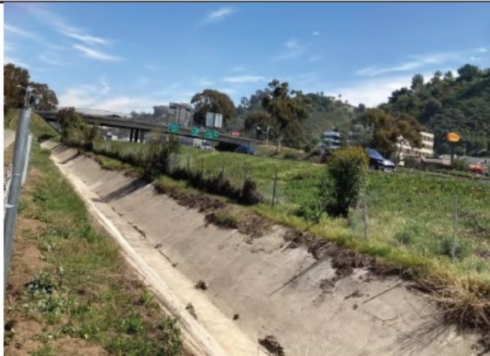
Post-Maintenance Photo Point 8: Looking east from the northern side of Camino del Rio 1 –vegetation and soil materials shown to be removed from channel, concrete repair shown (3/2/2022).
