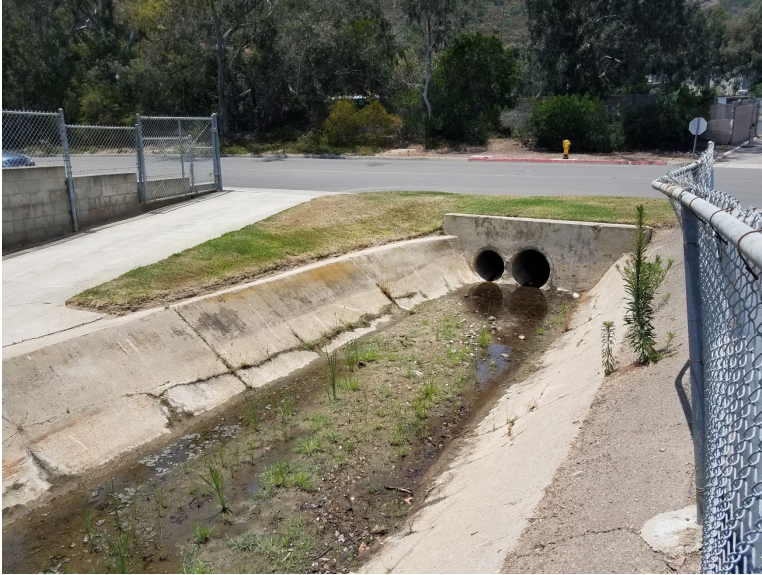
Flintkote premaintenance photo western terminus looking towards culverts and Flintkote Avenue (June 25, 2022)
