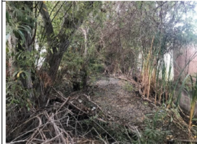
Pre-Maintenance - Photo 3: Pre-maintenance photo facing southwest from within the developed concrete lined channel looking at vegetation accumulated in the the Industrial 2 channel.
