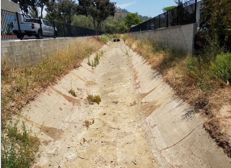
Flintkote pre-maintenance photo looking near Roselle Street east towards culverts that enter the Roselle channel, illustrating primarily silt and vegetation growth along the upper bank (June 25, 2022)
