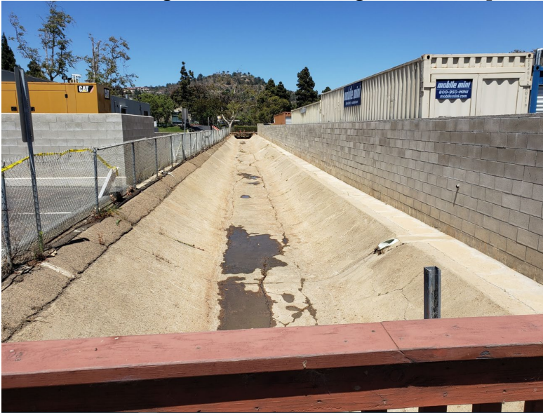
Flintkote post maintenance photo looking from mid-channel bridge crossing east towards Roselle Street (June 25, 2022)
