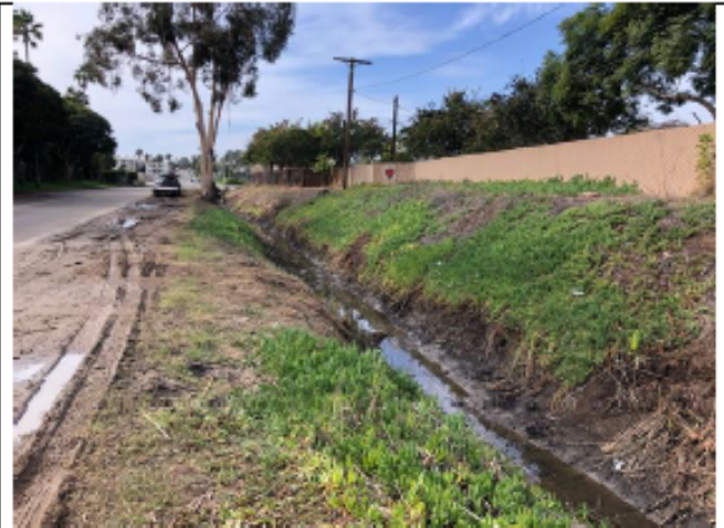
Photo Point 3 - Post-maintenance: photo looking northwest at where vegetation was removed from the PB-Olney 1 channel segment (12/10/2021).
