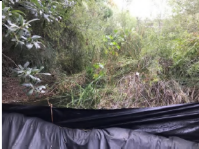
Roselle Pre-Maintenance - Photo 7: View of Roselle 1 (earthen channel), looking south. Silt fencing in view with non-native vegetation shown in background.
