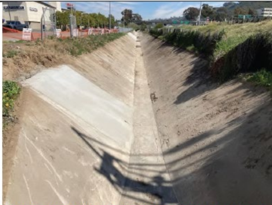
Post-Maintenance Photo Point 5: Looking east from western end of Camino del Rio 1. Vegetation had been removed from channel, concrete repair shown on left (3/2/2022).
