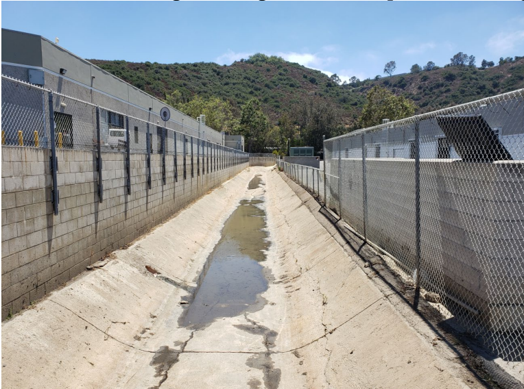
Flintkote post maintenance photo looking from mid-channel bridge crossing west towards Flintkote Avenue (June 25, 2022)
