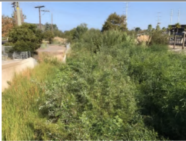
Roselle Pre-Maintenance - Photo 8: view showing both Roselle 1 & 2 taken from pedestrian crossing over Roselle 2, looking northwest. Thick vegetation shown to exist in channel.
