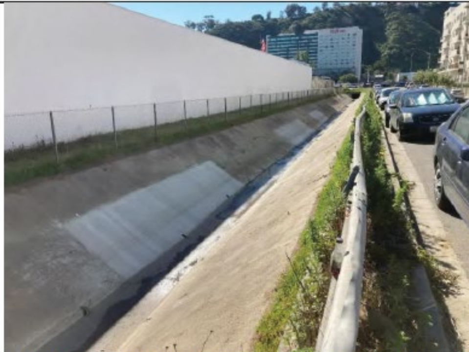
Post-Maintenance Photo Point 2: Looking southeast from the western edge of Camino del Arroyo 1 – vegetation shown to be removed from channel, concrete repair shown (3/2/2022).
