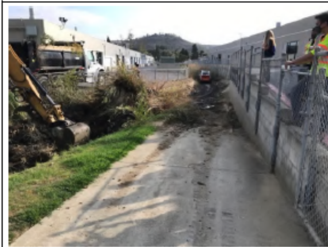
Flintkote Pre-Maintenance - Photo 1: view of Flintkote 1 looking northeast. Taken from western edge of project site. Thick vegetation shown in bed of channel. (September 16, 2021)
