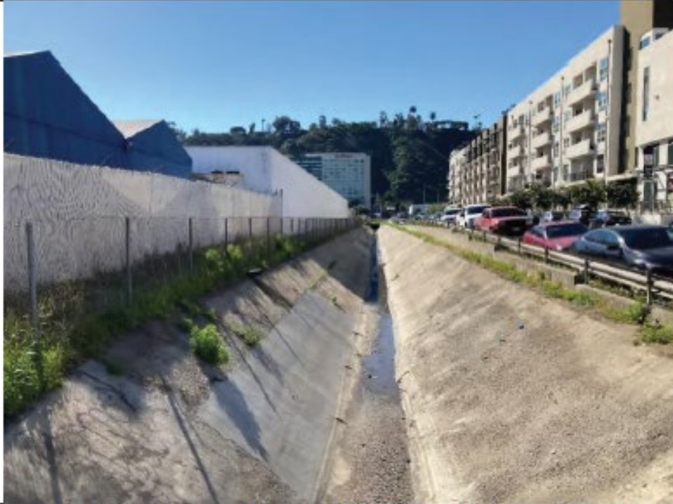
Post-Maintenance Photo Point 1: Looking south from the northern, downstream end of Camino del Arroyo-maintenance shown to be complete, concrete repair shown on left (3/2/22).
