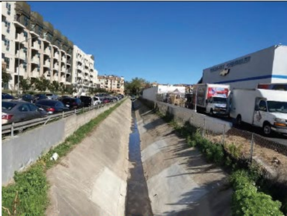
Post-Maintenance Photo Point 4: Looking north from the southern end of Camino del Arroyo 1 – vegetation shown to be removed from channel and concrete repair areas visible (3/2/2022).
