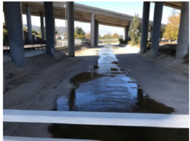
Roselle Post-Maintenance - Photo 10: view of Roselle 2 looking east from approximately the center of the channel showing vegetated and unvegetated sections of concrete-lining.
