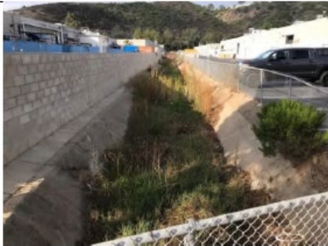
Flintkote Pre-Maintenance - Photo 4: View of Flintkote 1 looking south from Roselle Street crossing. Access area shown next to vegetated channel.
