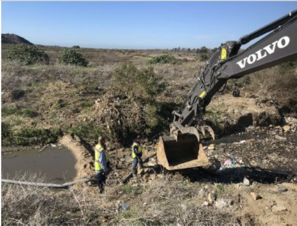
Photo 9: Dirt berm and pump being used to divert water flows away from the work area (1/04/2022).
