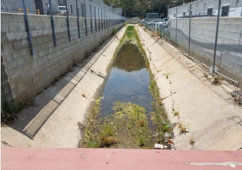
Flintkote pre-maintenance photo looking from mid-channel bridge crossing west towards Flintkote Avenue, illustrating standing water, silt, sparse and low growth vegetation (June 25, 2022)
