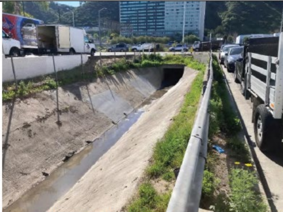
Post-Maintenance Photo Point 3: Looking south from the southern end of Camino del Arroyo 1 – vegetation shown to be removed from channel. Concrete repair areas shown. (3/2/2022).
