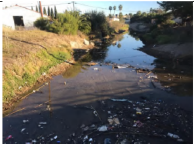
Photo – During-maintenance: Looking northeast from National Ave. bridge into the National 1 channel where water has inundated the maintenance area during high tides (November 15, 2021).
