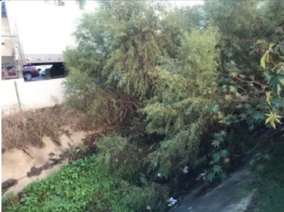
Pre-Maintenance Photo Point 3: Looking southeast from the southern end of Camino del Arroyo 1 – willow scrub/trees and vegetation shown within the channel at the start on maintenance (12/11/2021).
