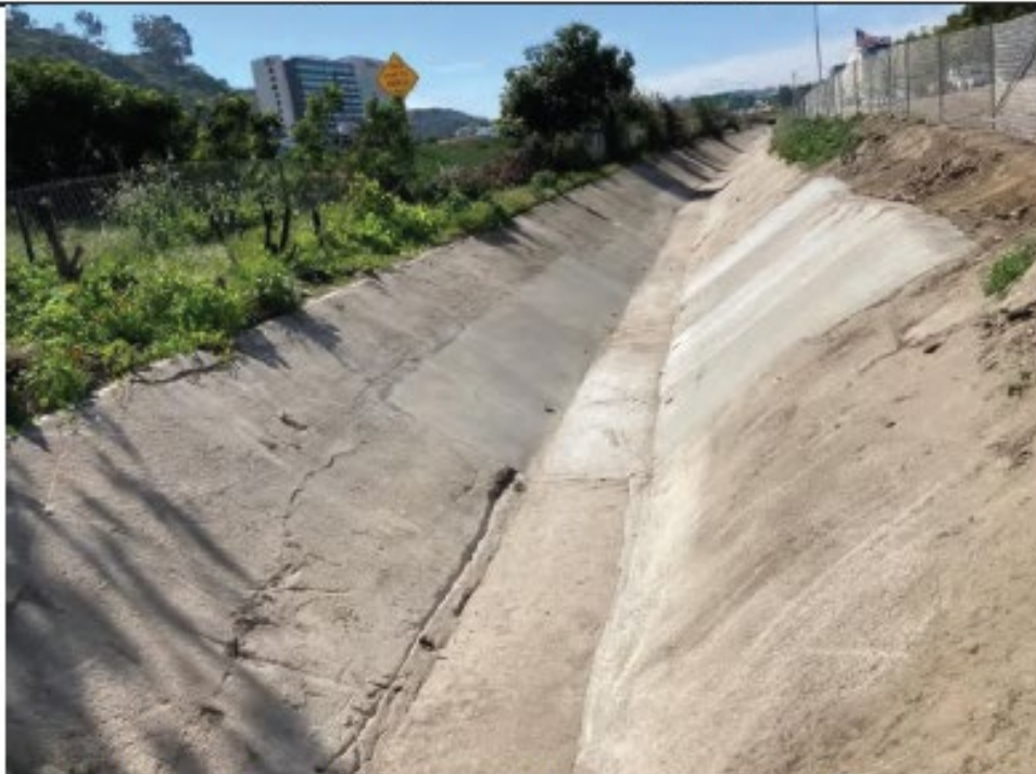
Post-Maintenance Photo Point 9: Looking southwest from the eastern, upstream end of Camino del Rio 1 where vegetation and material was removed. Concrete repair areas visible (3/2/2022).
