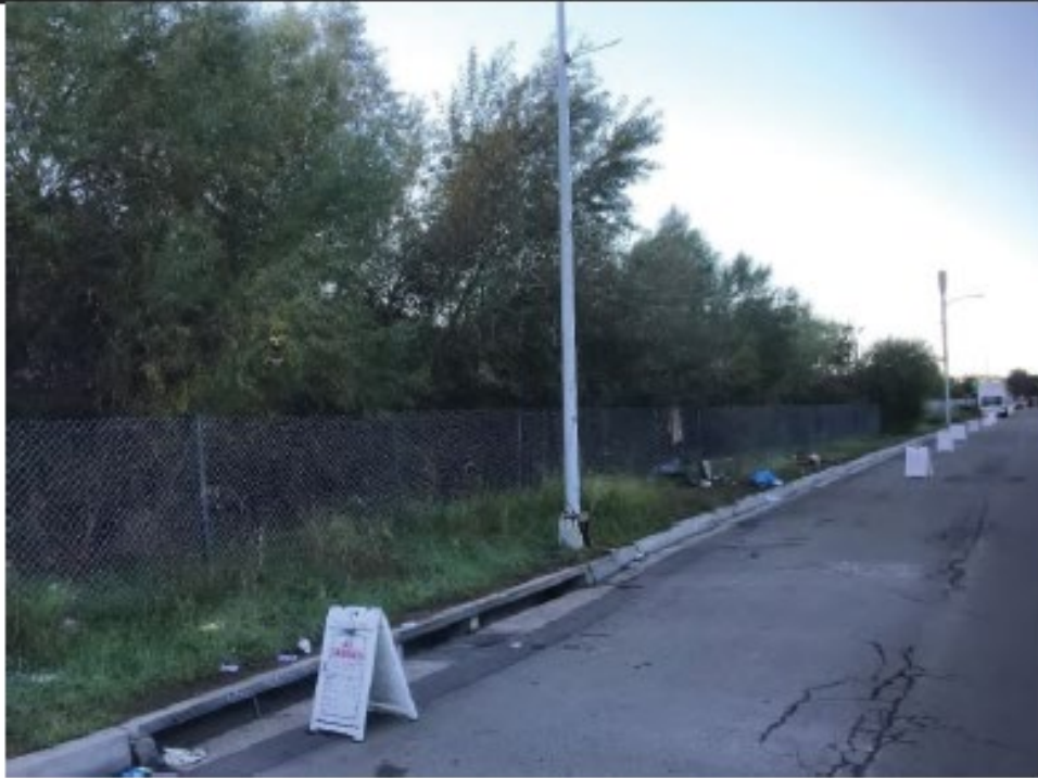
Pre-Maintenance Photo Point 7: Looking southwest from the northern side of Camino del Rio 1 at vegetation accumulated in the channel (12/11/2021).
