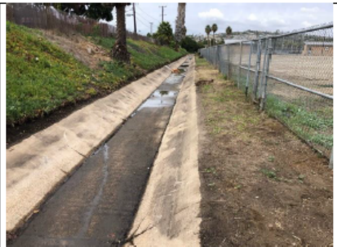
Photo Point 4 - Post-maintenance: photo looking northwest at where vegetation was removed from the MBHS 1 channel segment (12/10/2021).
