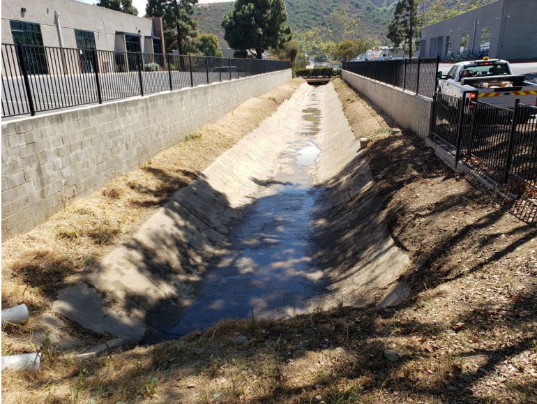
Flintkote post maintenance photo at the eastern terminus looking towards Roselle Street (June 25, 2022)
