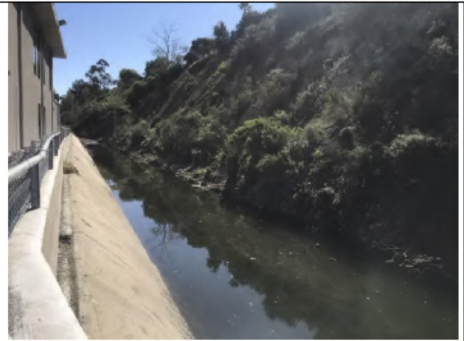
Photo Point 1 – Post-maintenance: Looking southwest within Alvarado 1 from the staging area at the channel cleared from excess vegetation (February 14, 2022).
