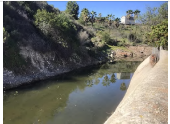
Photo Point 2 – Post-maintenance: Looking southwest within Alvarado 1 from the staging area at the channel cleared from vegetation and debris (February 14, 2022).
