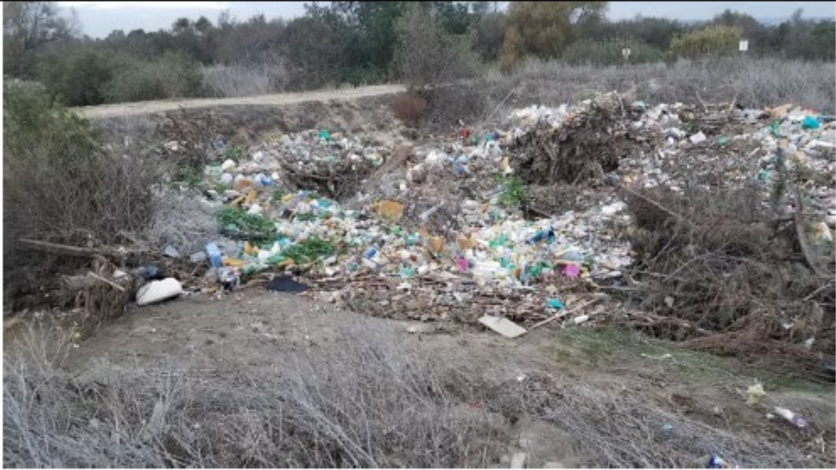
Photo 1: Pre-construction photo showing trash accumulation within the channel and blocking south side of Disney Bridge culverts (12/22/2021).
