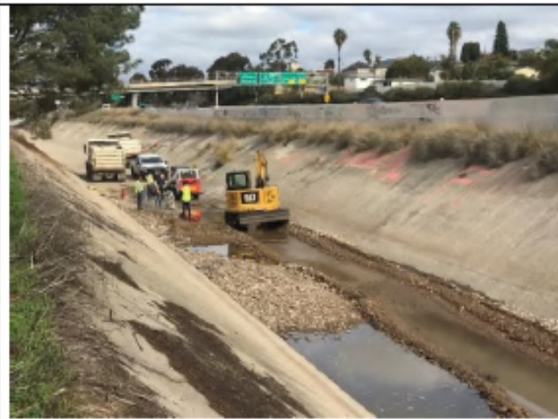
Photo – During-maintenance: Looking northeast within National 2 showing an excavator and dump trucks working within the concrete-lined channel (January 8, 2022).
