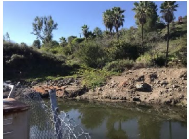
Photo Point 3 – Post-maintenance: Looking southwest within Alvarado 1 from the staging area at the banks of the channel cleared of invasive vegetation (February 14, 2022).
