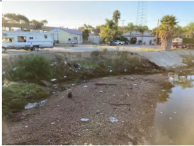
Photo Point 1 – Pre-Maintenance: Looking south within National 1 from the National Ave. bridge at material and trash accumulated within the channel (October 21, 2021).
