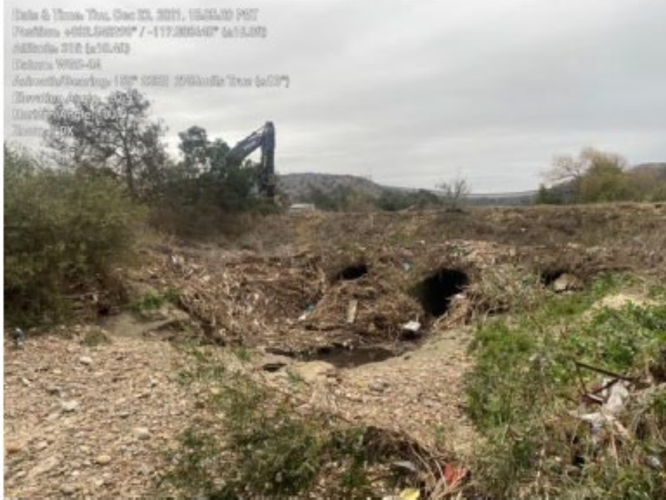
Photo 3: Pre-construction photo showing trash and debris blocking Disney Bridge culverts on the north side (12/23/2021).
