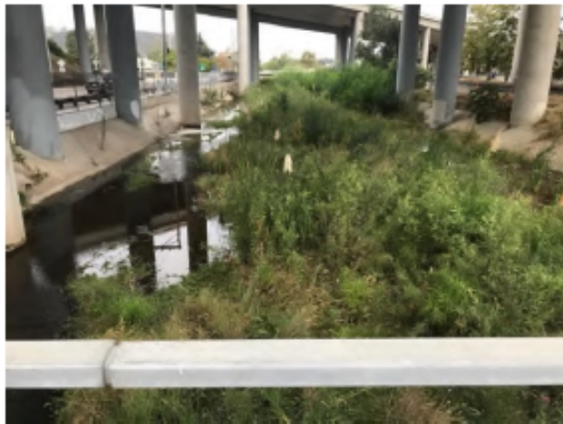
Roselle Pre-Maintenance - Photo 10: view of Roselle 2 taken from sidewalk that runs parallel to Sorrento Valley Blvd, near the intersection with Roselle Street. Thick vegetation shown to be present in channel.
