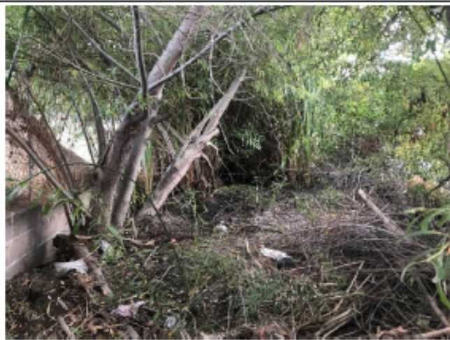
Pre-Maintenance - Photo 2: Pre-maintenance photo facing northeast from within the developed concrete lined channel looking at vegetation accumulated in the downstream end of the Industrial 2 channel maintenance area. (October 4, 2021)
