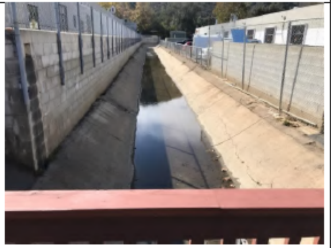
Flintkote Post-Maintenance - Photo 2: View of Flintkote 1, looking southwest towards the edge of the project site, taken from pedestrian footbridge. Maintenance activities shown to be complete (November 4, 2021)
