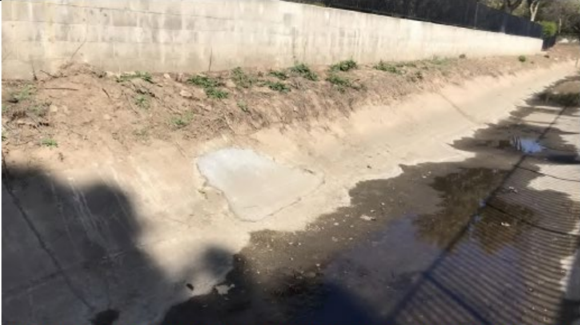
Flintkote Concrete Repair- Photo 5: View of concrete patching done within concrete-lined channel at Flintkote 1, looking northeast. (November 4, 2021)
