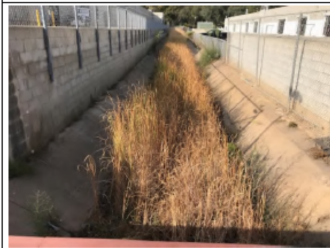
Flintkote Pre-Maintenance - Photo 2: View of Flintkote 1 looking south west towards the edge of the project site, taken from pedestrian footbridge. Vegetation shown in bed of channel. (September 16, 2021)
