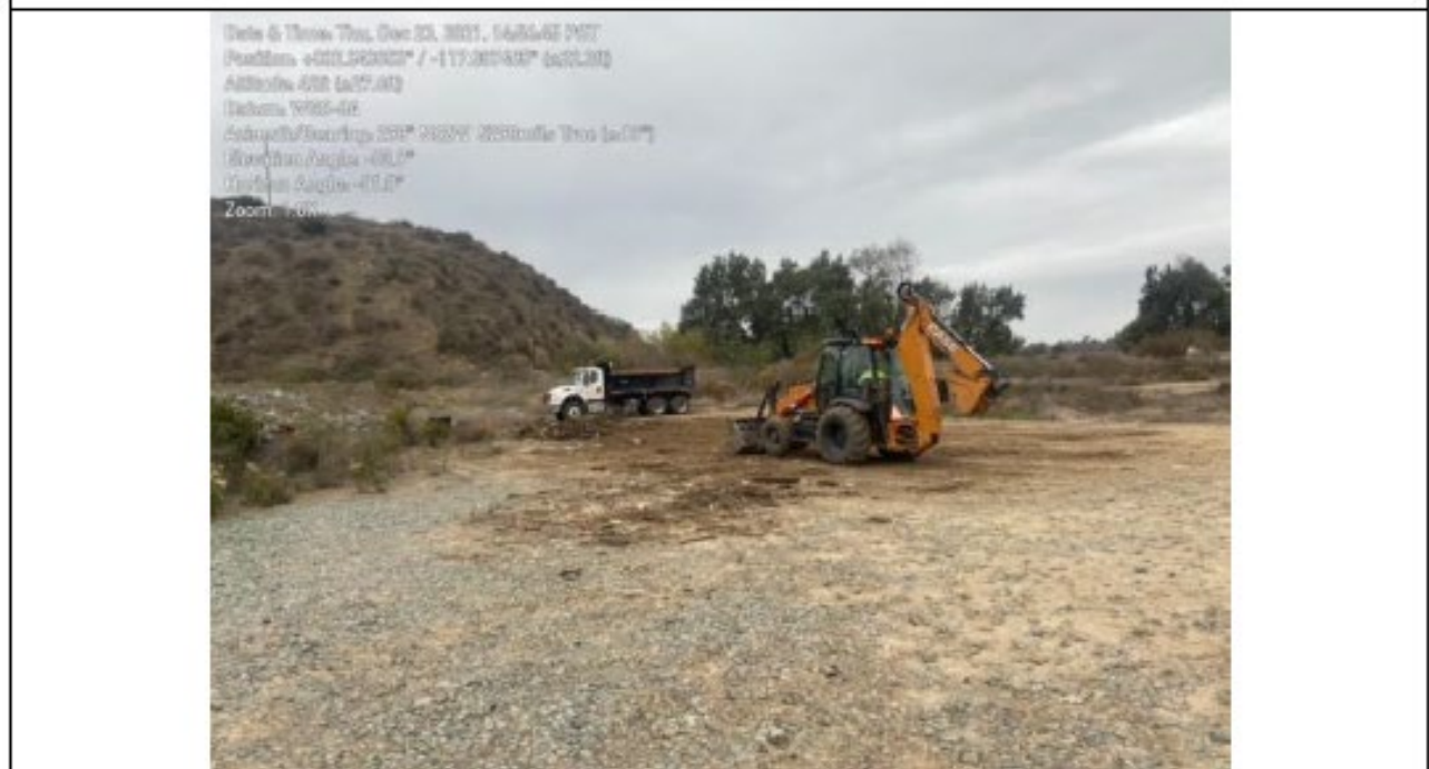
Photo 6: Debris from a stockpile in staging area being managed and loaded for removal by heavy machinery (12/23/2021).
