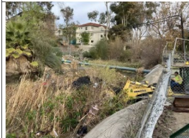
Photo Point 4 – During-maintenance: Looking northwest within Alvarado 1 from the staging area at overgrown vegetation and debris within the channel (January 31, 2022).
