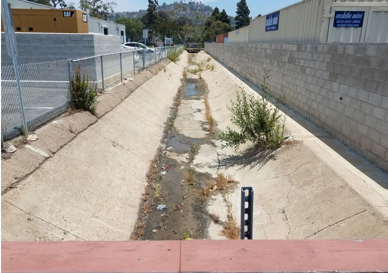
Flintkote premaintenance photo looking from mid-channel bridge crossing east towards Roselle Street, illustrating minor silt, standing water, and sparse vegetation growth (June 25, 2022)
