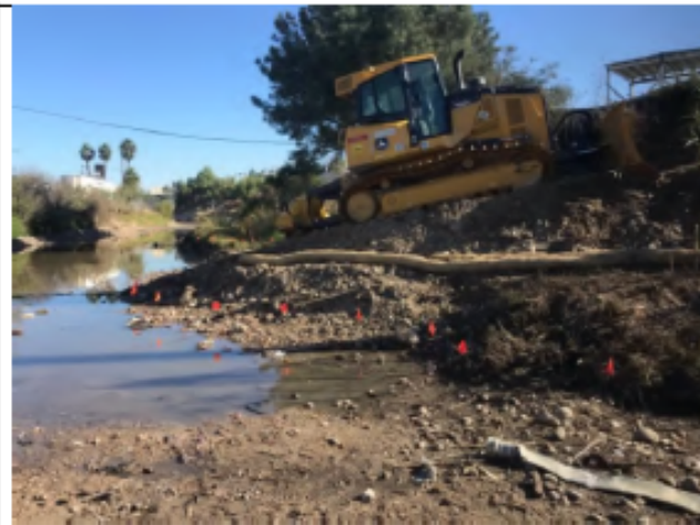
Photo – During-maintenance: Looking northeast within National 2 showing widened access ramp and sediment deposition as well demarcated disturbed coastal salt marsh (October 29, 2021).
