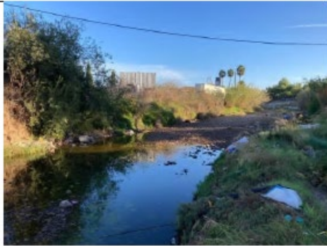
Photo Point 4 – Pre-maintenance: Looking north within National 1 from within the channel north of the National Ave. bridge towards National 2 prior to the start of maintenance (October 21, 2021).
