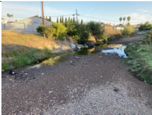
Photo Point 2 – Pre-maintenance: Looking north above National 1 from National Ave. bridge at vegetation and sediment/cobble accumulation within the channel (October 21, 2021).
