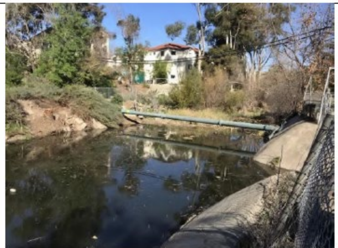
Photo Point 4 – Post-maintenance: Looking northwest within Alvarado 1 from the staging area at the channel cleared from vegetation and debris (February 14, 2022).
