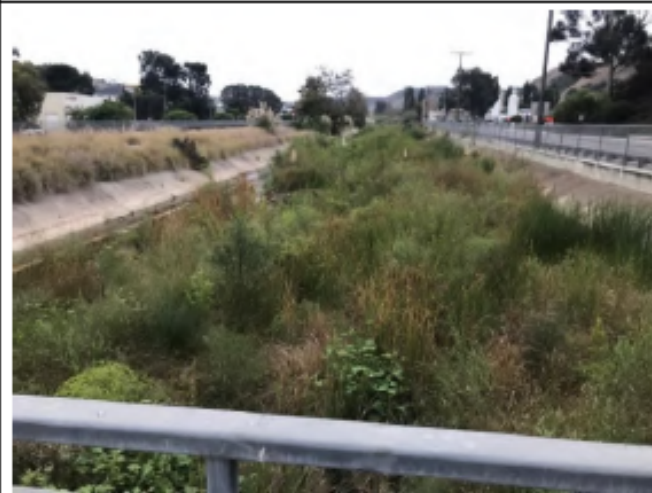
Roselle Pre-Maintenance - Photo 11: view of Roselle 2 looking east from approximately the center of the channel showing vegetated and unvegetated sections of concrete-lining.
