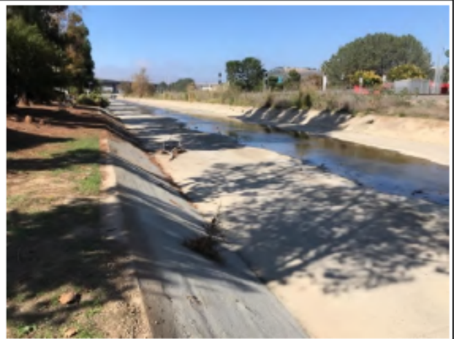
Roselle Post-Maintenance - Photo 12: view of Roselle 2 looking north from southern end of maintenance area. Maintenance activities shown to be complete.
