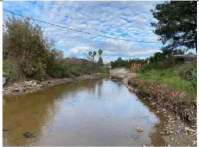
Photo Point 4 – Post-maintenance: Looking north within National 1 from within the channel north of the National Ave. bridge towards National 2 following completion of maintenance activities (January 17, 2022).
