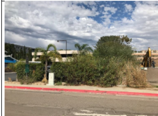
Pre-Maintenance - Photo Point 4: Pre-maintenance photo facing northeast from Sorrento Valley Road looking at vegetation accumulated in the downstream end of the Industrial 2 channel
