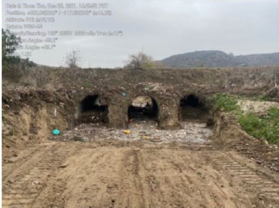
Photo 7: Looking south at Disney bridge culverts nearly cleared from trash and debris (12/23/2021).
