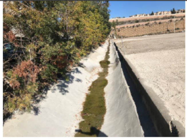
Post-Maintenance - Photo 2: Post-maintenance photo facing northeast from looking the cleared and repaired concrete lining within the Industrial 2 channel. (November 11, 2021)
