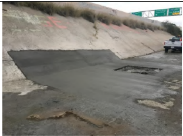
Photo - During-maintenance: Looking southeast within National 2 at the concrete repair location following concrete pour (January 13, 2022).
