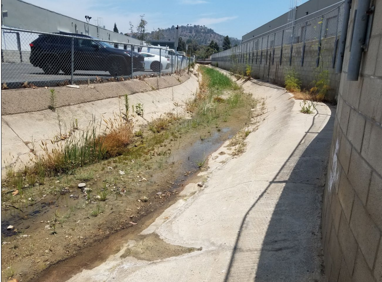
Flintkote pre-maintenance photo looking from the equipment access ramp on the western terminus east towards a mid-channel bridge crossing, illustrating silt, sparse and low growth vegetation (June 25, 2022)
