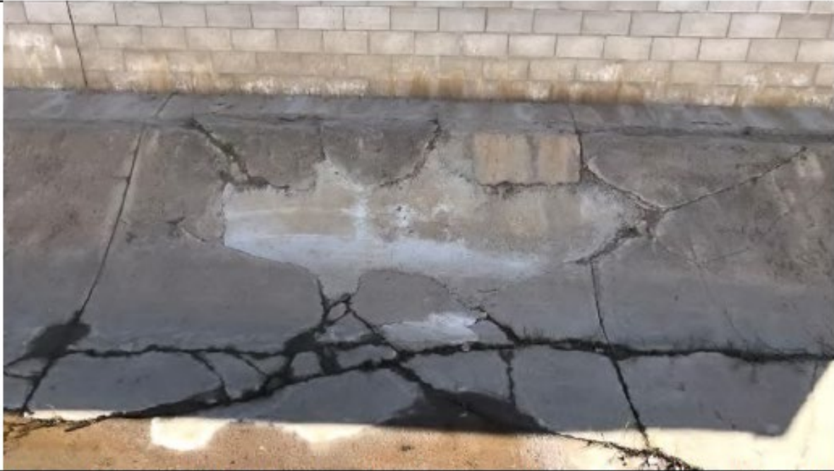
Flintkote Concrete Repair - Photo 3: View of concrete patching done within concrete-lined channel at Flintkote 1, looking south.
