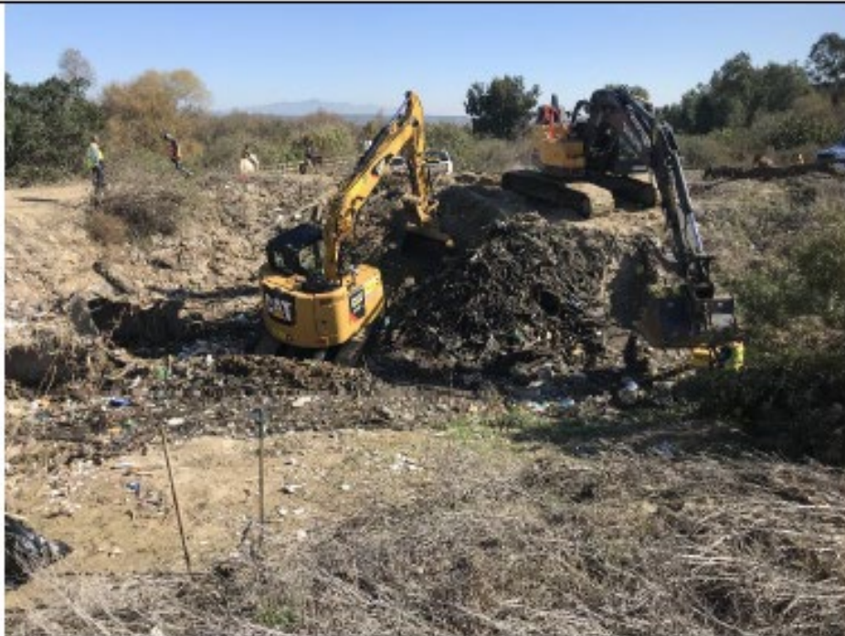
Photo 10: Excavators used to continue the removal of trash, debris, and detritus from the channel (1/04/2022).
