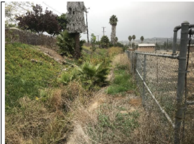
Photo Point 4 - Pre-maintenance: photo looking northwest at dense vegetation within the MBHS 1 channel segment (12/1/2021).
