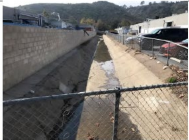
Flintkote Post-Maintenance - Photo 4: View of Flintkote 1 looking south from Roselle Street crossing. Vegetation removal shown to be completed.
