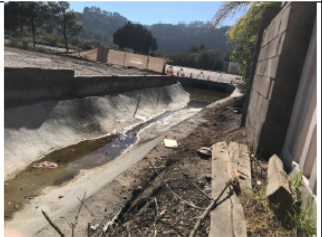
Post-Maintenance - Photo 3: Post-maintenance photo facing southwest looking towards the culvert inlet under Sorrento Valley Boulevard at the cleared and repaired concrete lining within the Industrial 2 channel.
