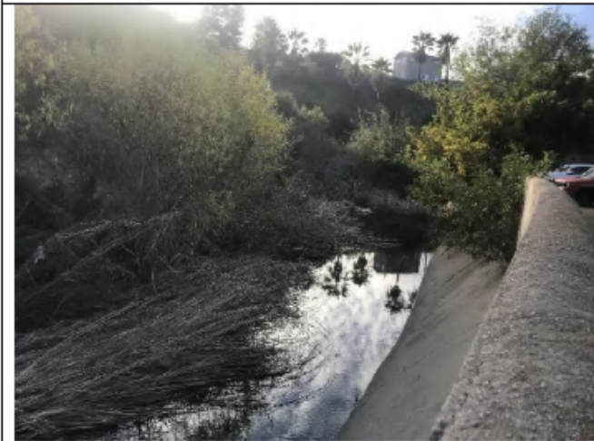
Photo Point 2 – Pre-maintenance: Looking southwest within Alvarado 1 from the staging area at overgrown vegetation within the channel (January 26, 2022).
