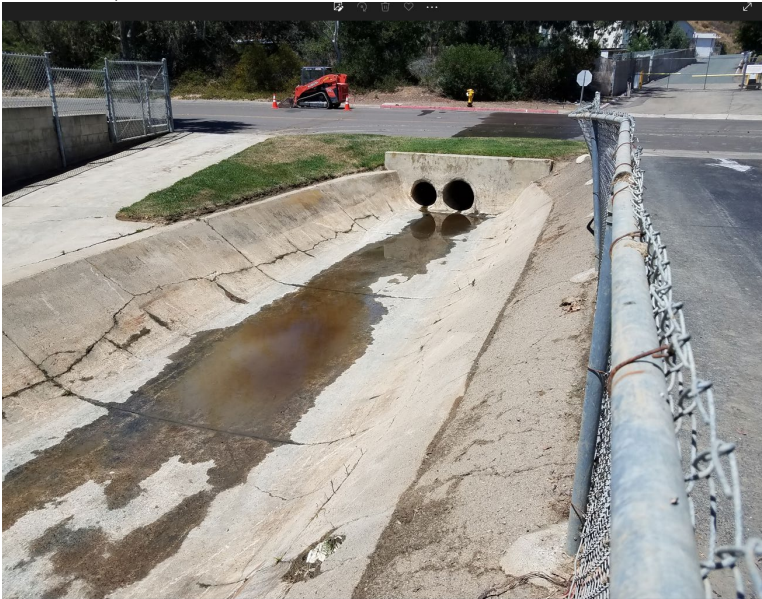
Flintkote post maintenance photo western terminus looking towards culverts and Flintkote Avenue (June 25, 2022)
