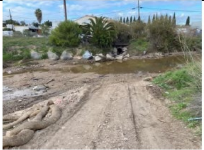
Photo Point 3 – Post-maintenance: Looking northwest at access ramp following completion of channel maintenance activities (January 17, 2022).
