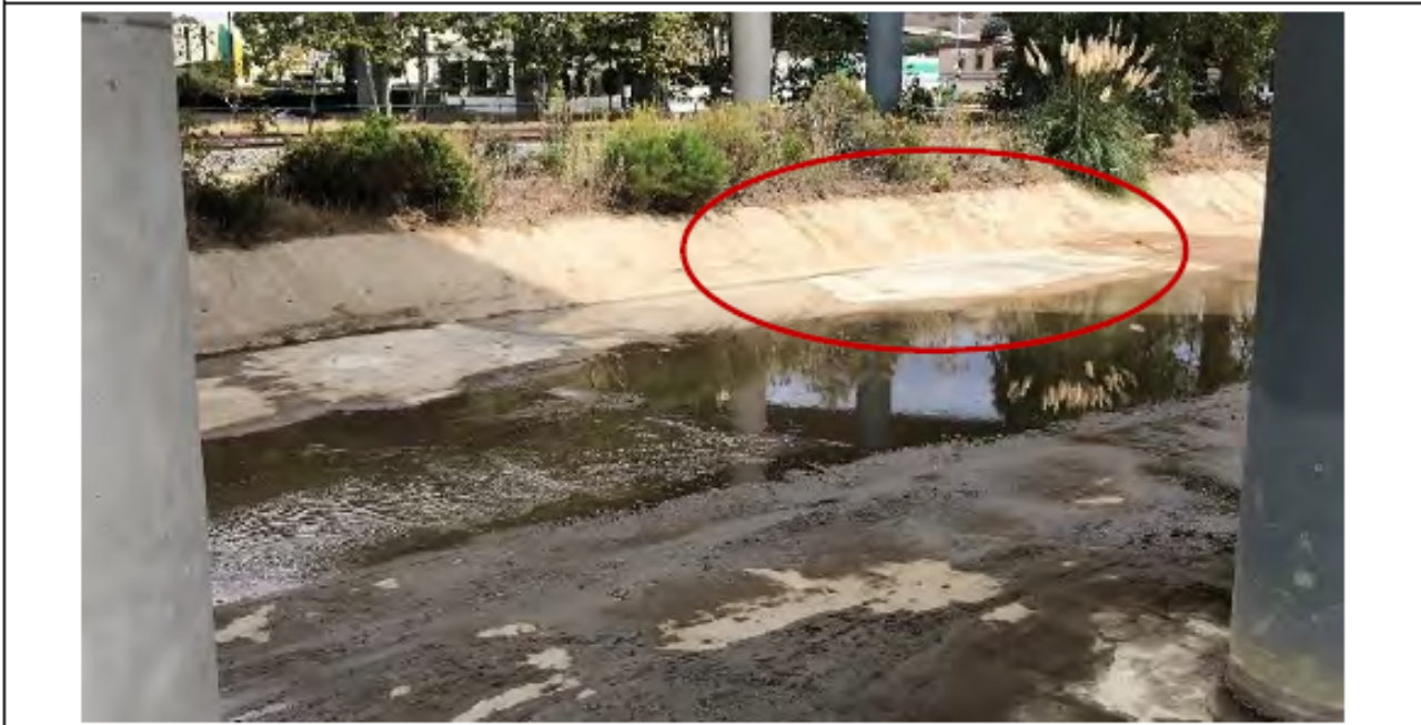
Roselle Concrete Repair- Photo 9: View of minor concrete repair area (circled in red) completed within concrete-lined channel at Roselle 2, looking southeast.
