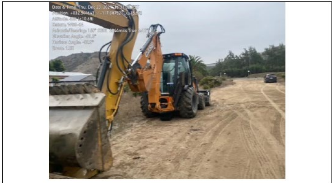
Photo 5: Drip pans placed under equipment parked in staging area (12/23/2021).
