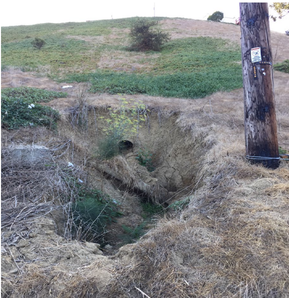
Photo 17: Facing uphill showing failed pipe and resulting sink hole directly next to the SDG&E transmission pole. Photo taken September 30, 2020.
