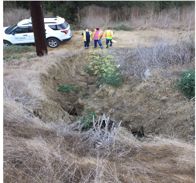
Photo 18: Facing downhill showing failed pipe section and resulting sink hole. Taken September 30, 2020.
