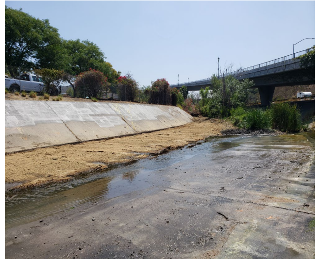
Photo 10: Facing upstream of the Mission Gorge 3 channel segment showing earth section of channel with vegetation removed and coir mat installed. Taken June 29, 2021.
