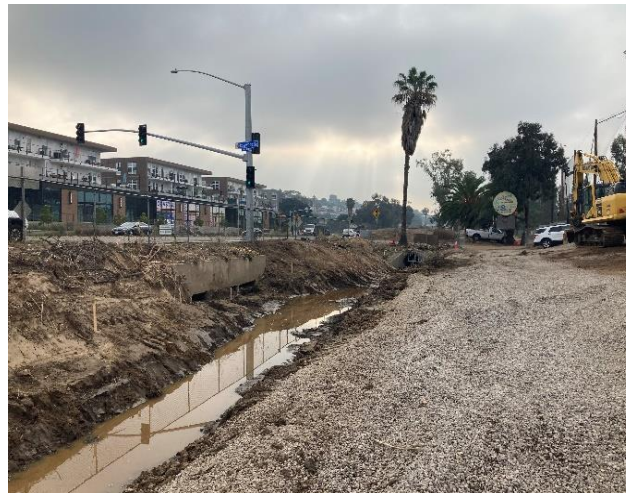
Photo 4: Facing downstream of the Mission Bay Drive-1 Channel following completion of maintenance. Taken February 8, 2021.
