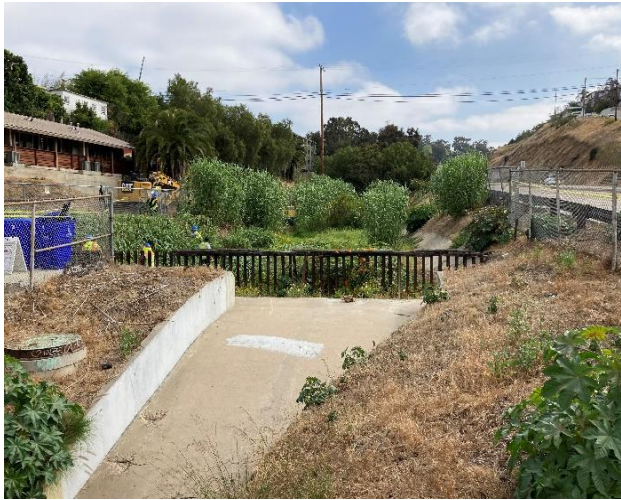
Photo 13: At the downstream section of the Washington 1 segment pre-maintenance with the concrete lined spillway that leads into the downstream culvert in the foreground. Taken June 1, 2021.
