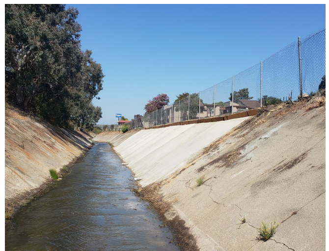
Photo 12: Facing downstream of the Mission Gorge 4 channel segment following completion of maintenance and new concrete panels. Taken September 2, 2021.
