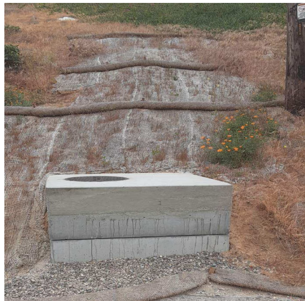
Photo 20: Facing uphill showing re-established slope grade, new Type-A cleanout, and post-maintenance erosion controls. Taken May 20, 2021.
