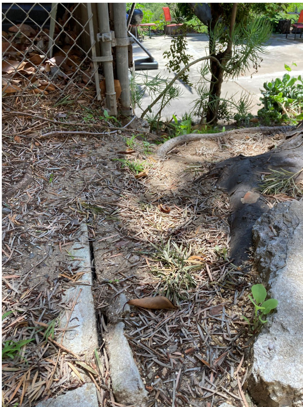
SOIL SEPARATION: TREE HAS SHIFTED
