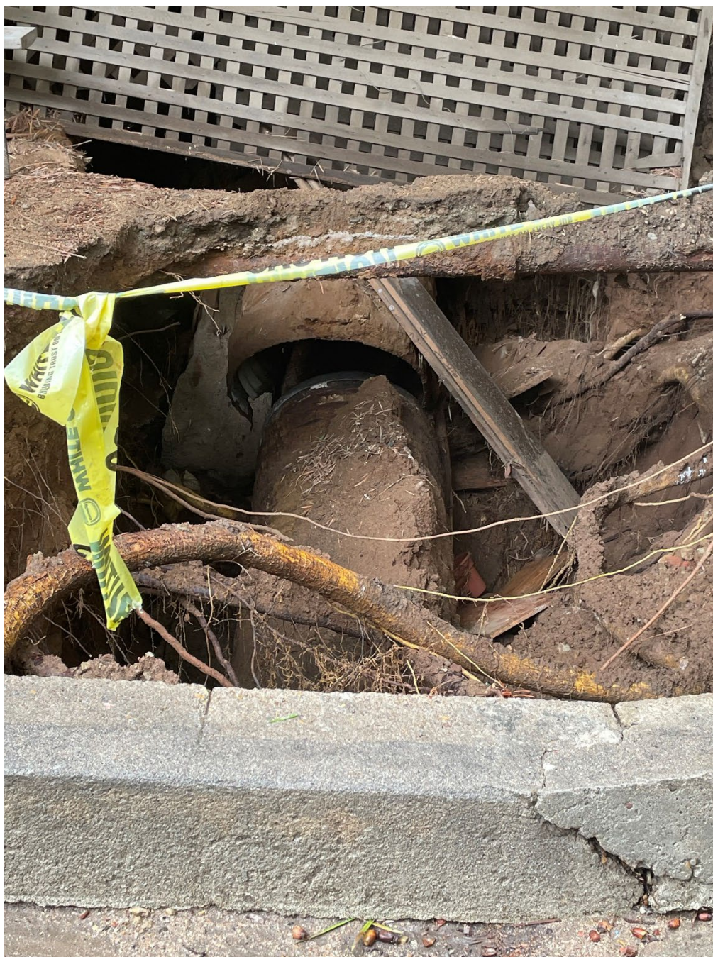
SINKHOLE: DISCONNECTED PIPE
