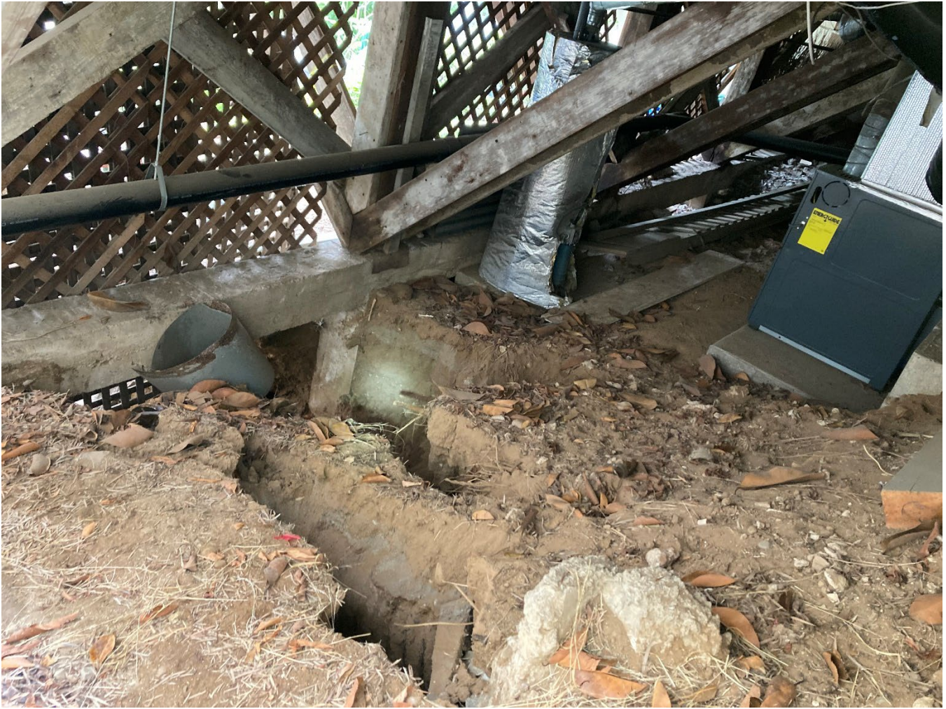
SINKHOLE: CONCRETE SUPPORT BEING IMPACTED
