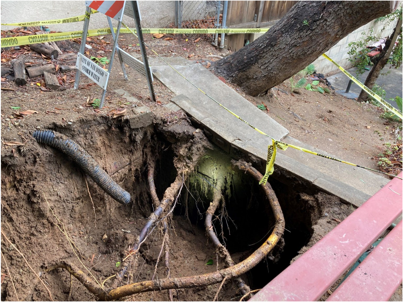
SINKHOLE: VISIBLE FAILURE AND UNDERMINED TREE
