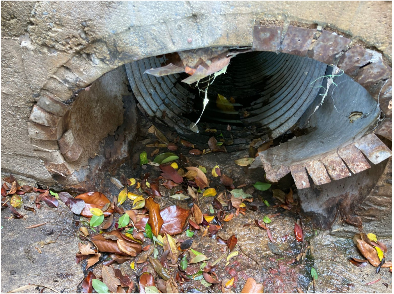
INLET: PIPE DISCONNECT AND VOIDS
