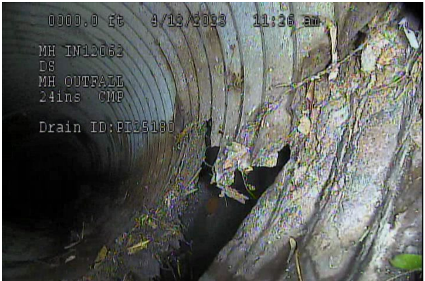
CCTV: HOLE IN PIPE
