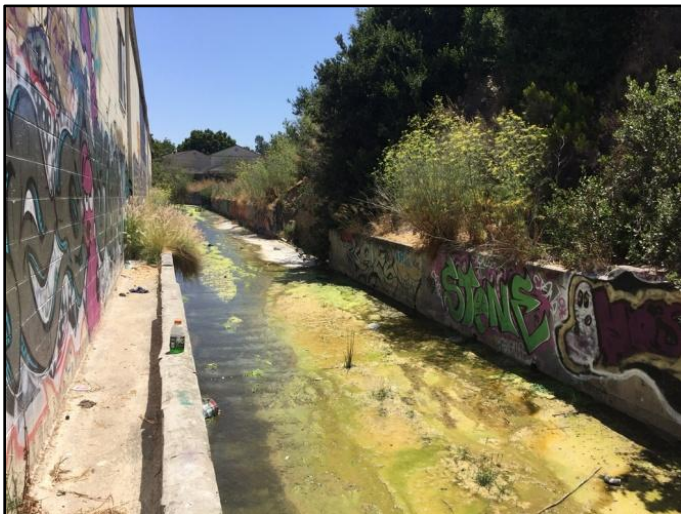
Figure 1: July 2017, looking upstream; missing sidewalk and eroded bank at center
