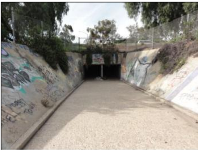
Figure 1: March 2016, looking downstream towards 7-foot wide by 6-foot tall double RCB culvert. Note clean channel.
