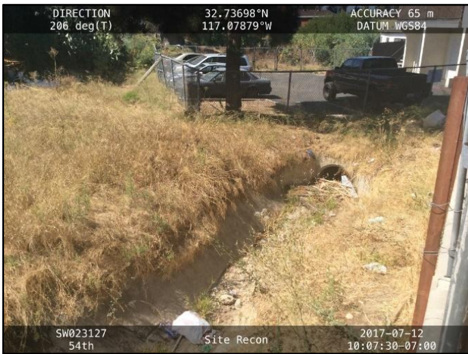
Figure 1: July 2017, looking downstream towards the culvert; conveys flows beneath parking lot, then discharges back into ditch
