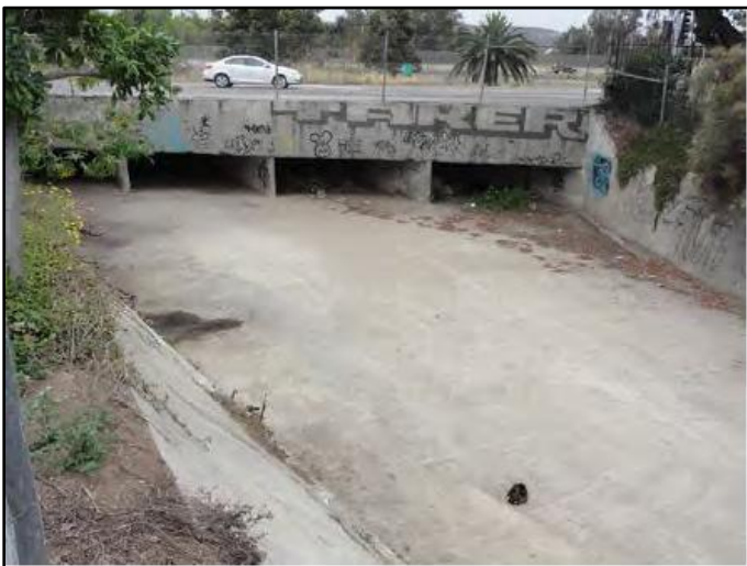
Figure 1: April 2015, looking downstream at entrance to quadruple 12-foot-wide by 4-foot-high RCB culvert beneath West San Ysidro Boulevard
