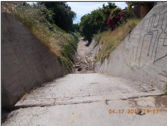
Figure 1: April 2017, looking downstream at second drop structure and sediment accumulated at bottom of structure
