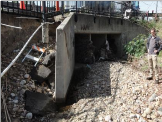
Figure 1: February 2017, standing along east bank of segment, looking southwest at erosion behind east wing wall at downstream end
