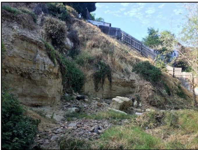
Figure 1: August 2017, looking downstream toward channel bank failure/erosion
