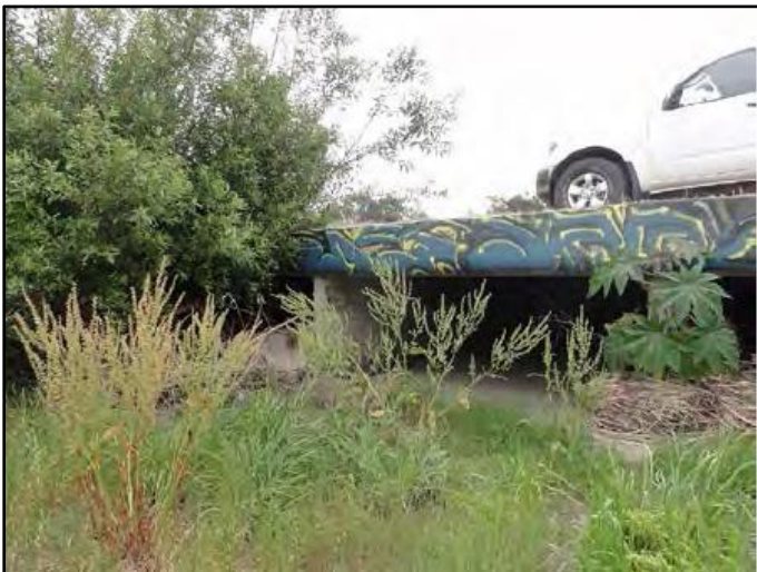
Figure 1: April 2015, looking downstream at entrance to quadruple 12-foot-wide by 4-foot-high RCB culvert beneath Interstate 5
