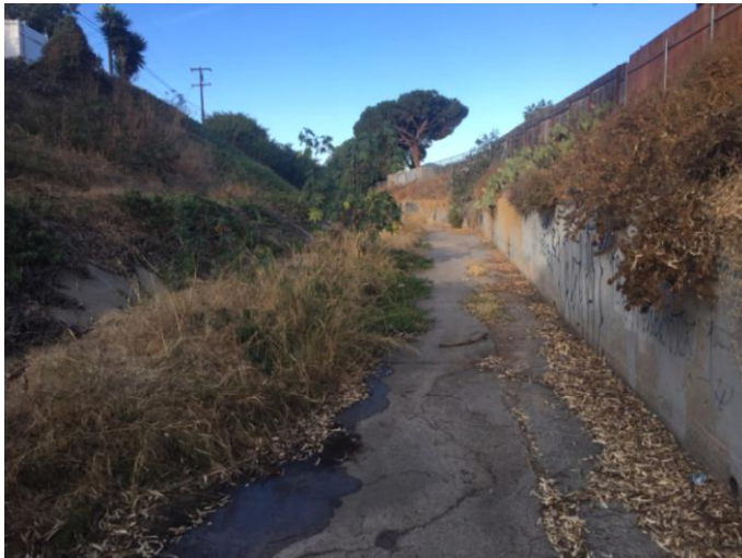
Figure 1: April 2017, looking downstream at accumulated sediment and debris in concrete channel
