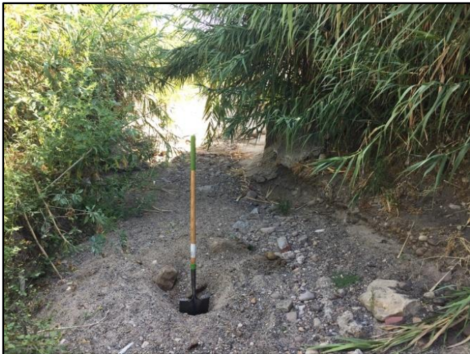
Figure 1: August 2017, looking upstream just after transition from concrete to earthen lining; deep sediment observed
