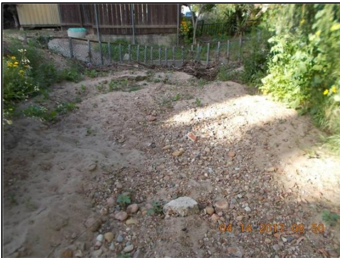
Figure 1: April 2017, looking downstream at sediment and debris accumulated at debris fence
