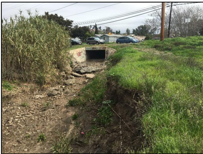
Figure 1: April 2016, upstream of 10-foot-wide by 5-foot-high RCB culvert beneath 69th Street facing west
