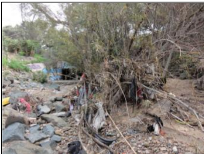
Figure 1: March 2016, looking upstream at the vegetation and displaced riprap downstream of the double 7-foot wide by 6-foot tall RCB culvert
