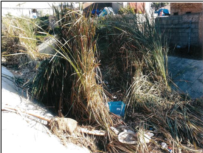
Figure 1: December 2014, looking upstream at dense vegetation, and sediment and debris within ditch
