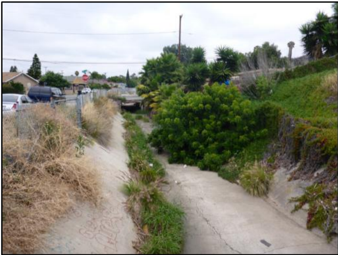
Figure 1: May 2015, looking upstream from double 9-foot-wide by 5-foot-tall RCB culvert at 40th Street
