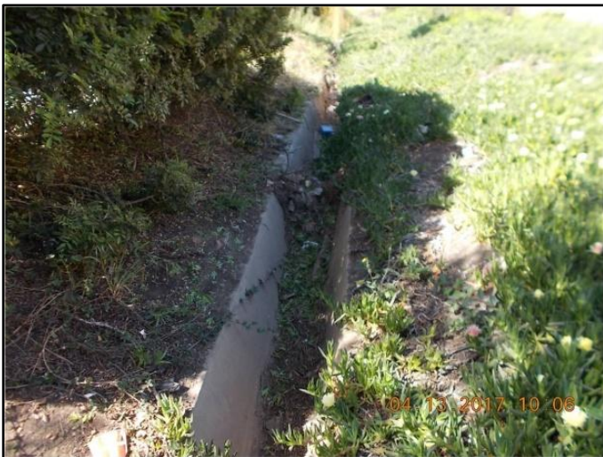
Figure 1: April 2017, looking downstream at sediment, debris and overhanging vegetation upstream of Outer 1 and Outer 2 junction
