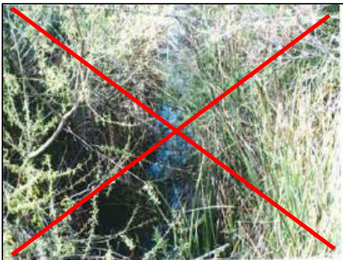
Figure 1: March 2013, heavily vegetated channel bottom near the downstream end of the facility group
