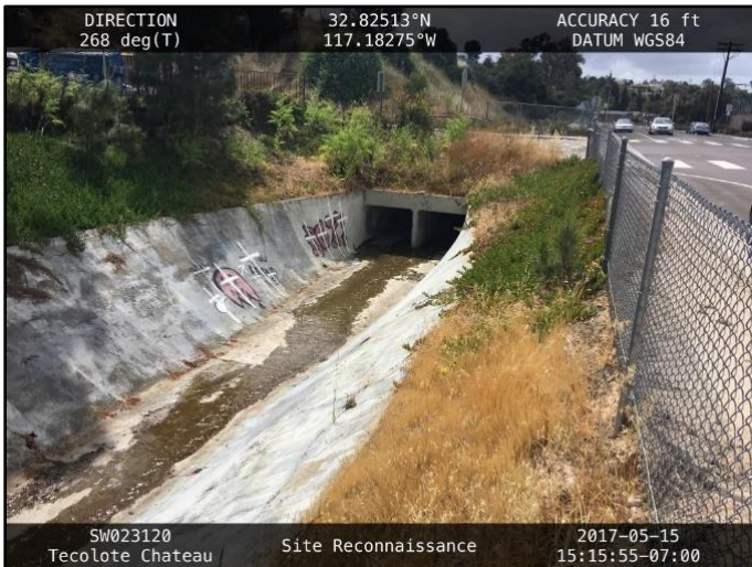
Figure 1: May 2017, upstream of double 5-foot-wide by 4-foot-high RCB culvert beneath Derrick Drive
