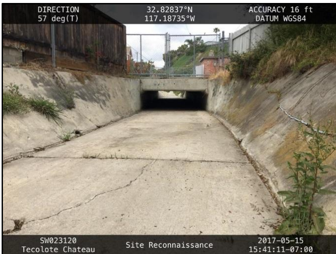
Figure 1: May 2017, downstream of 10-foot-wide by 3-foot-high RCB culvert beneath Chateau Drive
