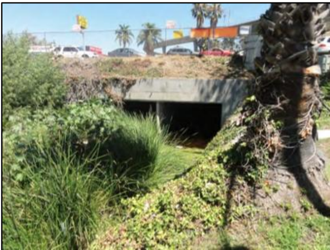
Figure 1: August 2014, looking upstream at the triple 12-foot-wide by 8-foot-tall RCB culvert beneath Fairmount Avenue
