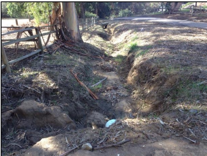
Figure 1: April 2017, representative of light weeds in the channel segment
