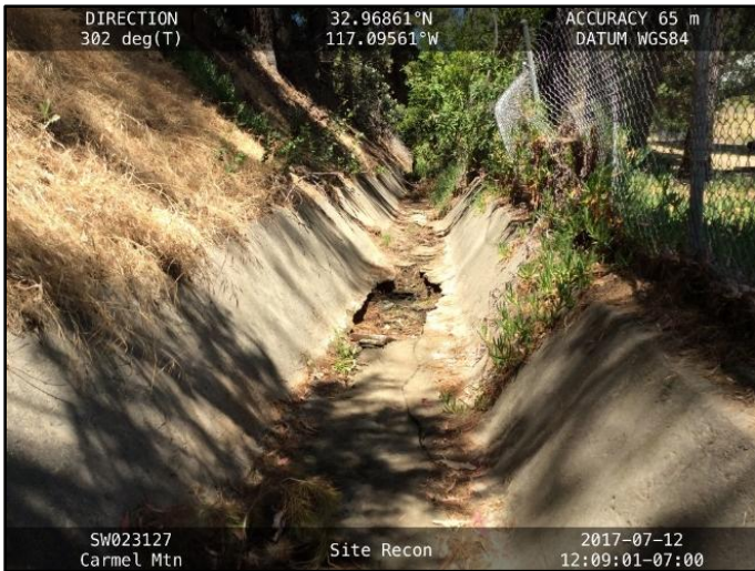
Figure 1: July 2017, photo depicts failure of gunite bottom of ditch, looking upstream
