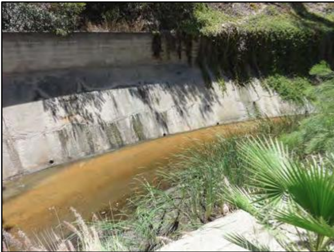
Figure 1: August 2014, from north side of the channel within 100% concrete portion of channel at 90-degree bend, looking downstream
