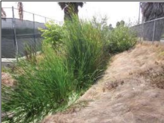
Figure 1: September 2013, at upstream end of segment, just downstream of 27-inch-diameter RCP and headwall. High density of vegetation observed, and concrete ditch is not visible.
