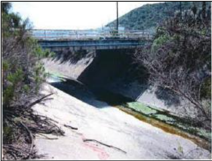
Figure 1: March 2013, looking downstream towards access road bridge near the upstream limit of concrete channel lining
