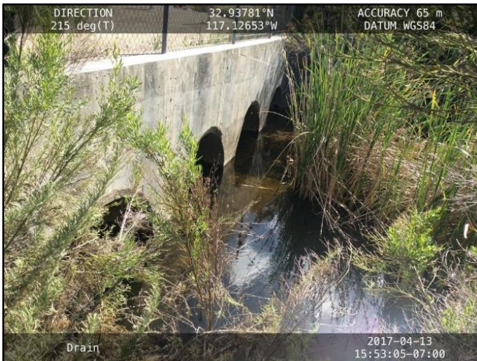
Figure 1: April 2017, looking upstream at quadruple-barrel 6-foot-diameter RCP storm drain outlet at Mercy Road
