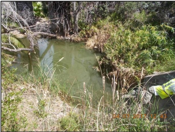
Figure 1: April 2017, looking downstream at scour pool at channel outfall
