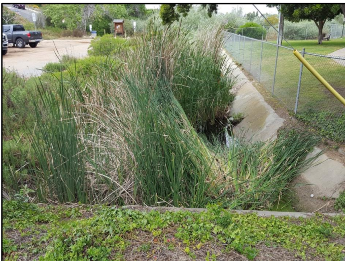
Figure 1: April 2017, looking downstream over headwall and 48-inch-diameter and 30-inch-diameter diameter RCP culvert outlet
