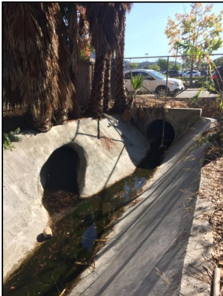
Figure 1: September 2017, facing the upstream end of the segment, at the location of the recent concrete lining repair work
