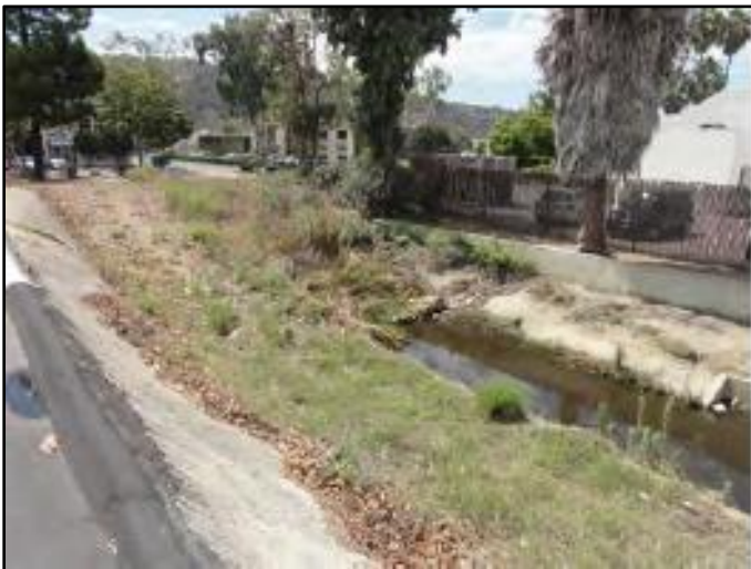
Figure 1: August 2014, looking downstream at double-barrel 57-inch RCP culvert entrance; downstream end of facility group
