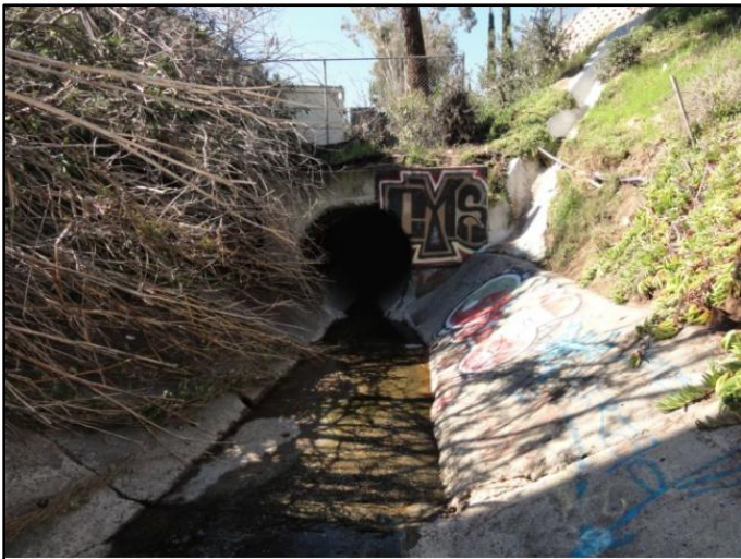
Figure 1: November 2016, facing downstream end of facility group; towards 60-inch-diameter RCP culvert beneath the Collwood Villas Apartments and Collwood Boulevard
