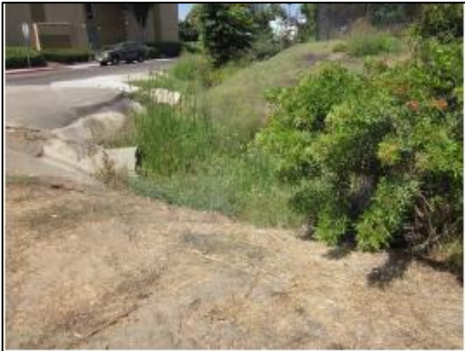
Figure 1: September 2013, downstream end looking east. High vegetation density and growth were observed
