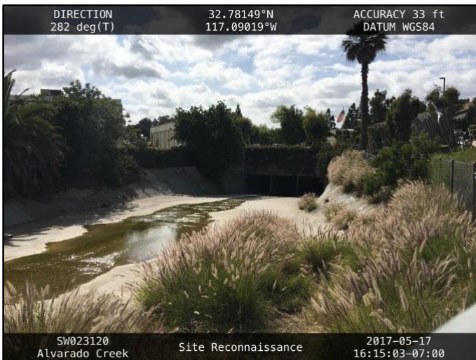
Figure 1: May 2017, looking at the downstream end of segment, towards the triple 9-foot wide by 8-foot high RCB culvert beneath Mission Gorge Place
