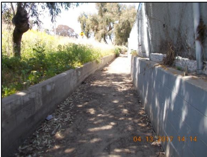
Figure 1: April 2017, looking downstream at sediment and debris at upstream end of concrete ditch
