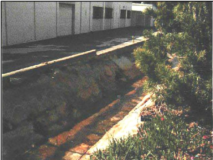
Figure 1: October 2009, looking downstream at concrete segment
