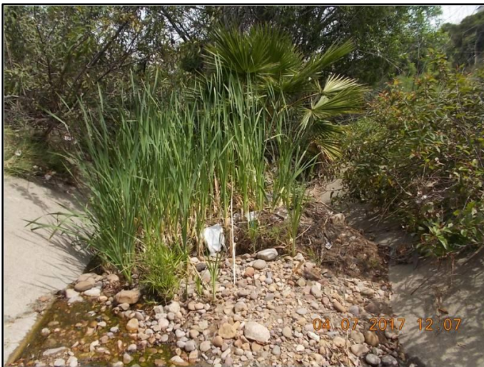
Figure 1: April 2017, looking downstream at sediment, debris and vegetation in concrete ditch
