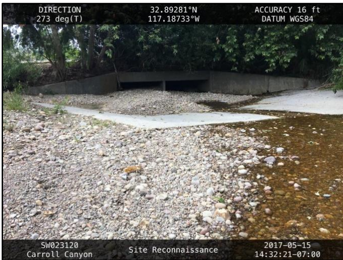
Figure 1: May 2017, sediment and cobbles accumulated on concrete inlet apron upstream of the culvert
