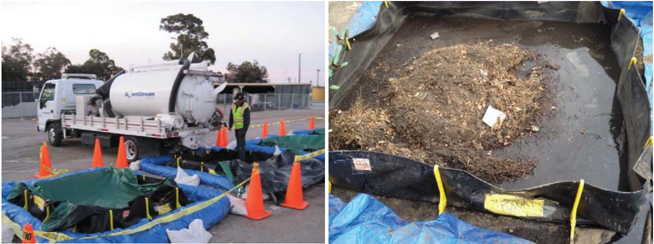
Figure 8. Delivery of materials to the containment berms for storing and drying before sampling and analysis.
