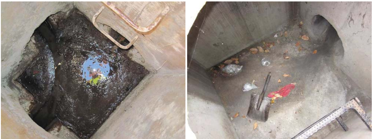
Figure 29. Catch basin interiors, showing deep and shallow sumps in Tecolote and San Ysidro.
