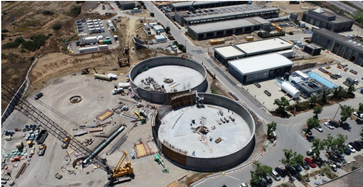
North City Pure Water Facility
