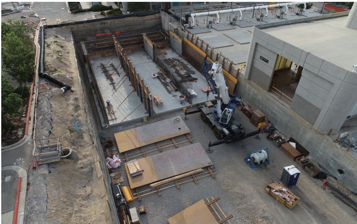
North City Water Reclamation plant
