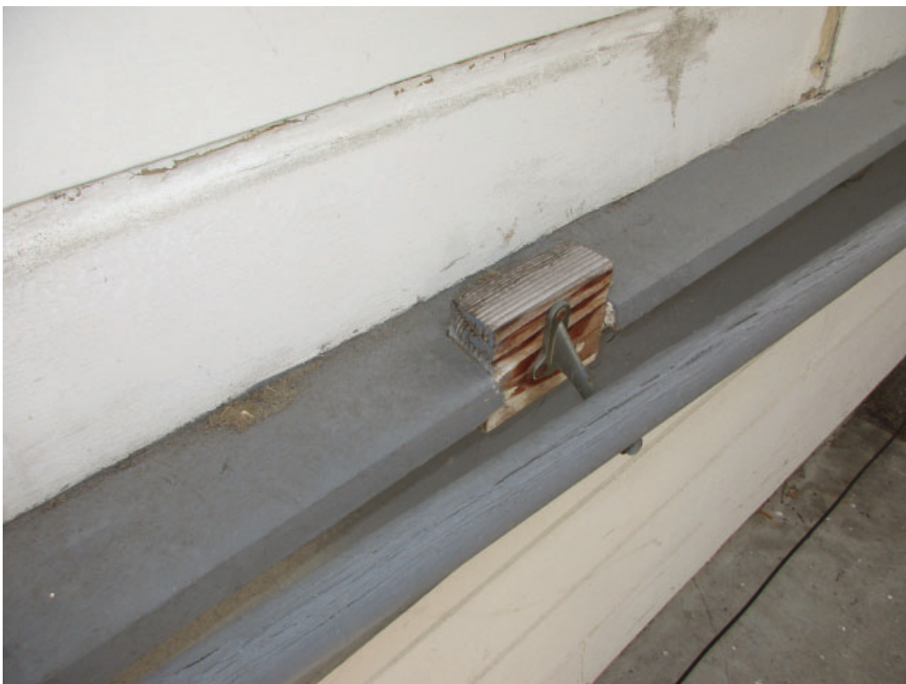
Figure 3-14: Detail photo showing the impact to the base trim boards from the accessibility ramp handrail attachments.
