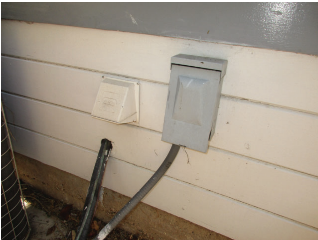
Figure 3-18: Detail photo showing some of the utility equipment installed at the base of the north facade.
