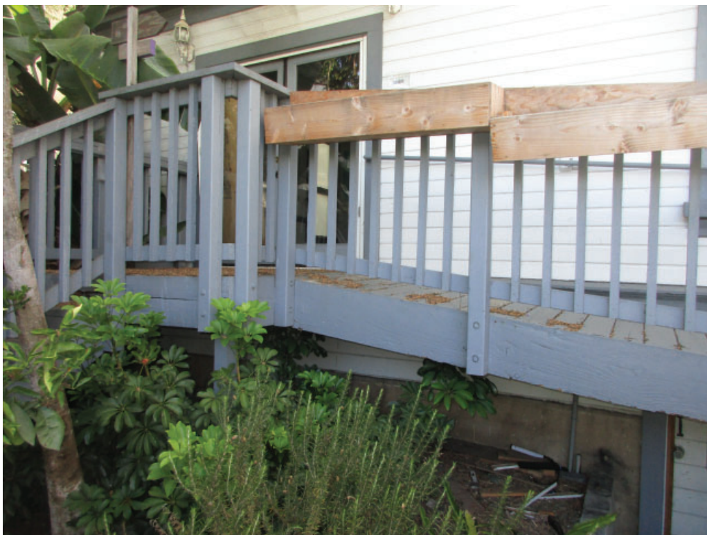
Figure 3-16: Looking northeast at the non-historic OSB board ramp and landing with wood railing. The wood components are termite damaged.
