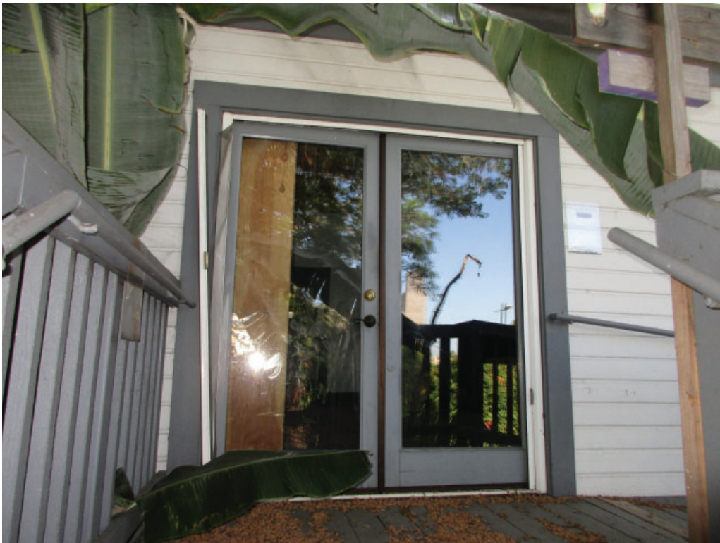
Figure 3-17: Looking east at the west facade showing the non-historic pair of wood french doors.
